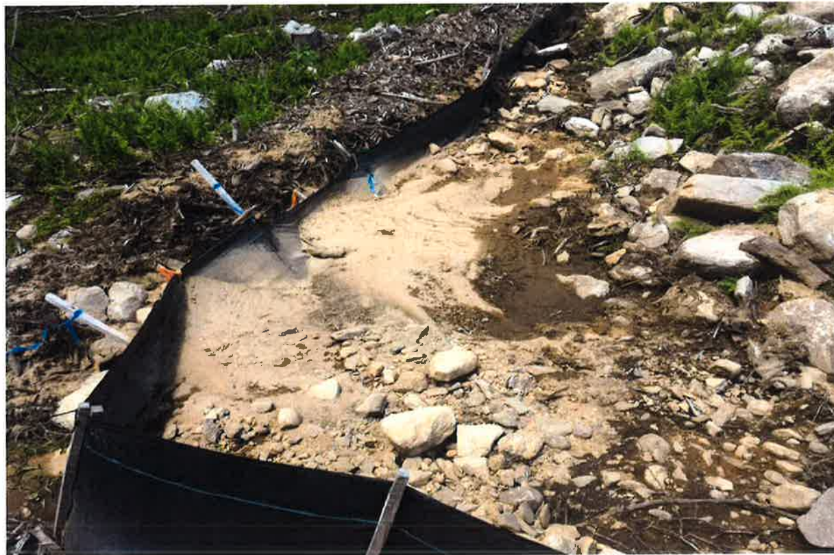
Photo 6: View of CA #12 (silt build-up), looking west.
