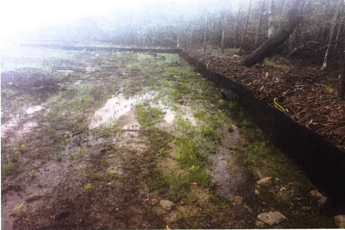
Photo 3: View of silt fence edge on western project boundary looking south.
