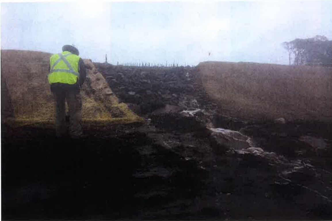
Photo 6: View of TO-8 outfall looking east.
