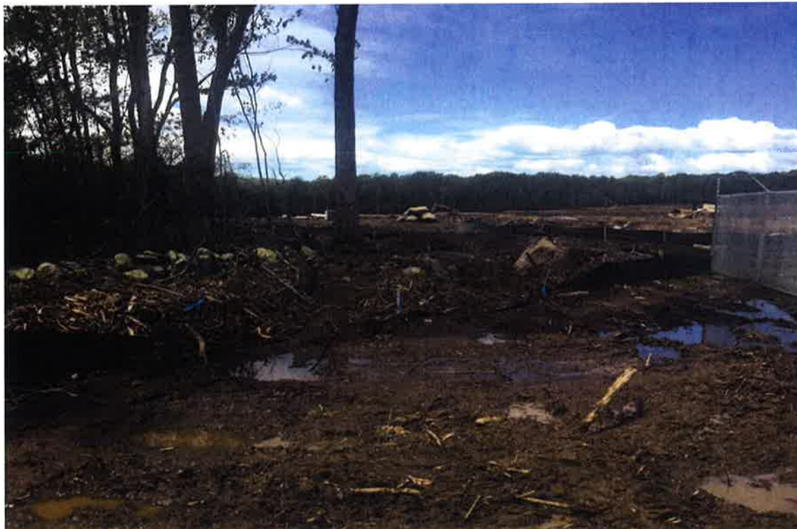
Photo 2: View of silt fence needing repair (CA #11), looking north.
