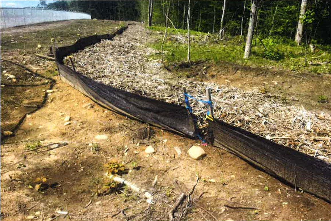
Photo 3: View of gap in silt fence (CA #11) requiring repair.
