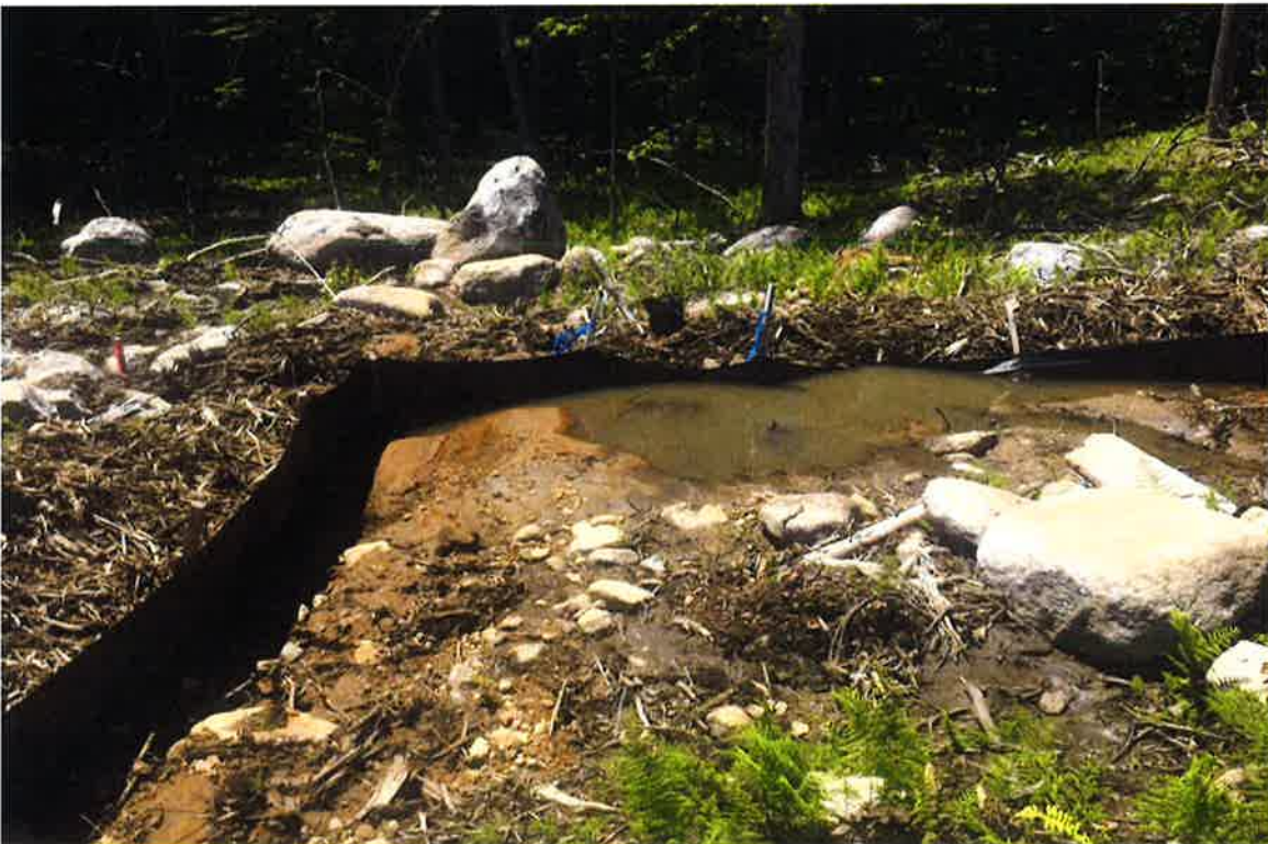
Photo 4: View of continued problem area (CA #8) in northwest corner looking west.
