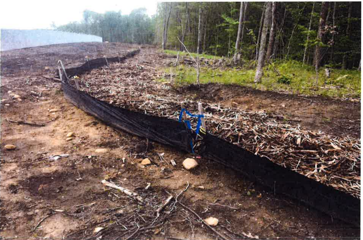
Photo 6: View of gap in silt fence (CA #11), looking northeast.
