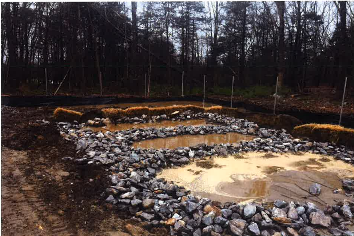
Photo 4: View of drainage from SB-3 build-up in southwest corner of project area, looking south.
