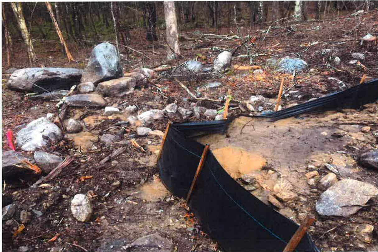
Photo 2: View of CA #8, breach in silt fence looking west.
