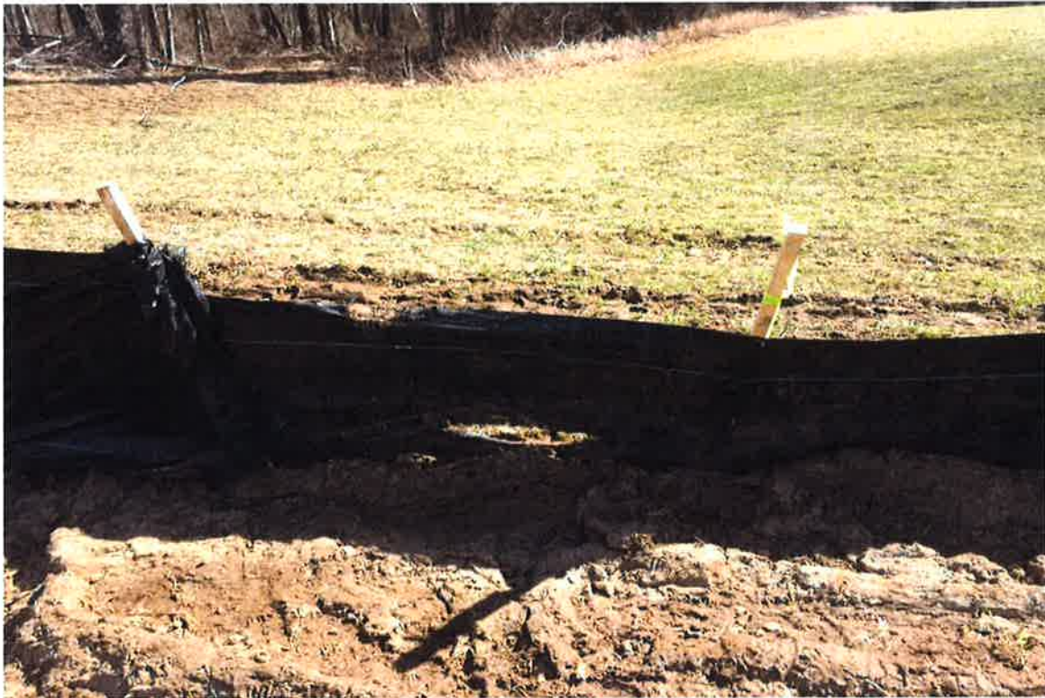
Photo 3: View of CA#4 silt fence hole/gap.
