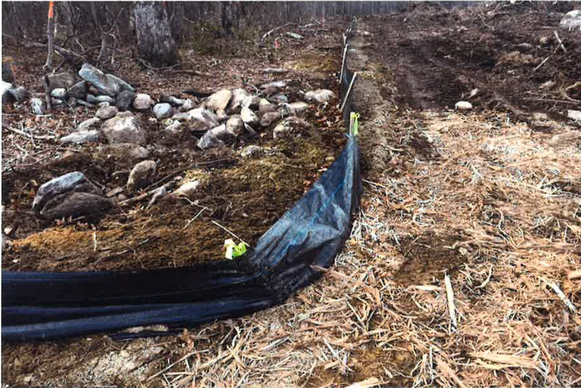
Photo 5: View of CA #6, area of insufficient silt fence height due to sagging.
