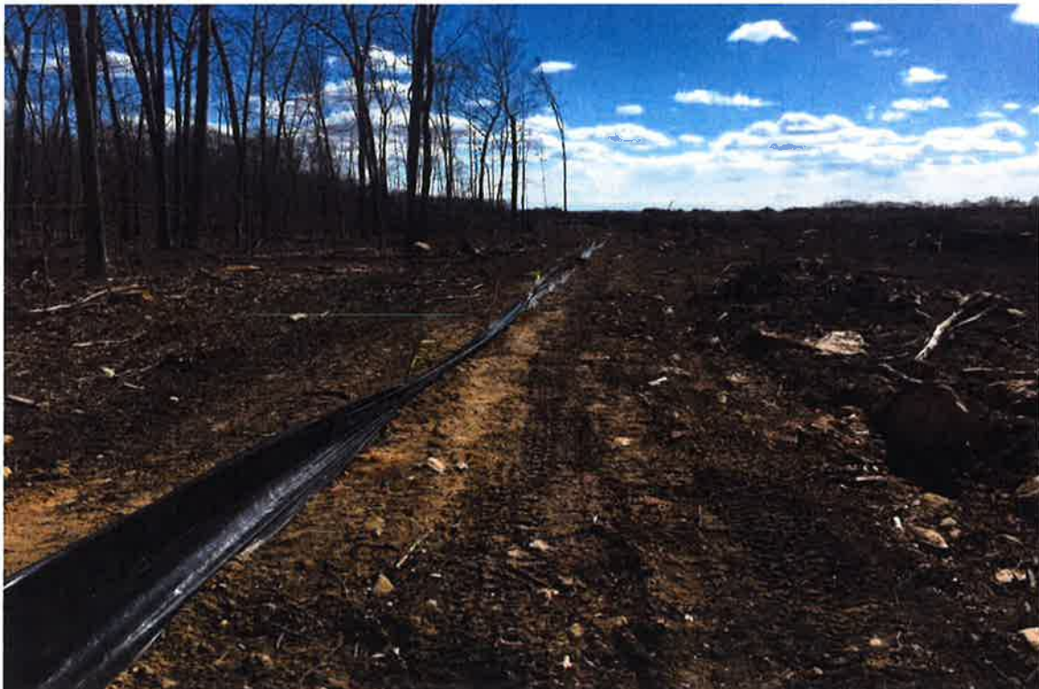
Photo 6: View of CA #6 where silt fence has ripped off staking.
