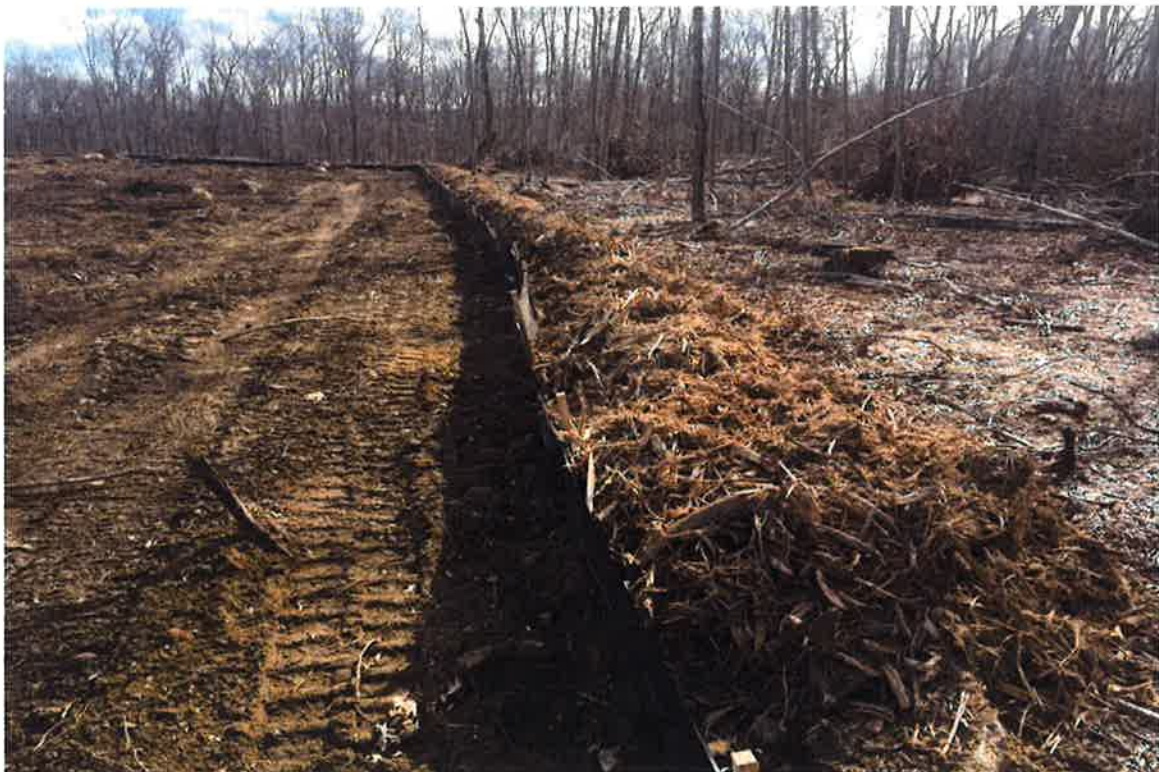
Photo 4: View of CA#5 where wood chips backing silt fence are pushed up to top. Wood chips need to be pushed away from silt fence to not allow herpetofauna migration into work zone.
