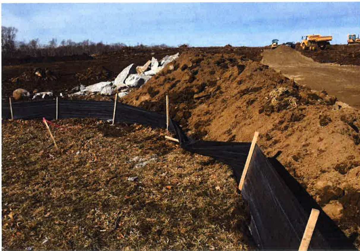
Photo 8: View of CA# 3 silt fence knocked over requiring repair.
