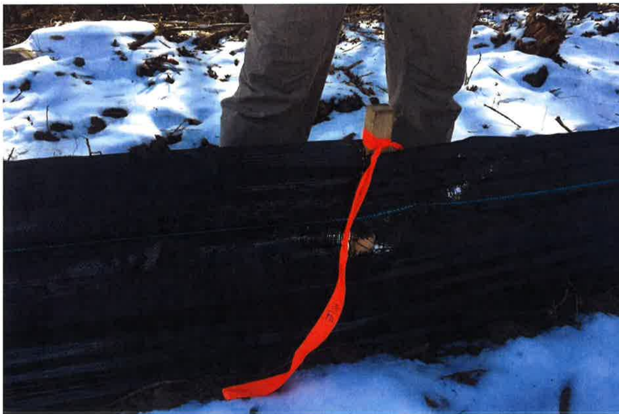
Photo 6: View of CA# 2 silt fence gap (flagged for repair).
