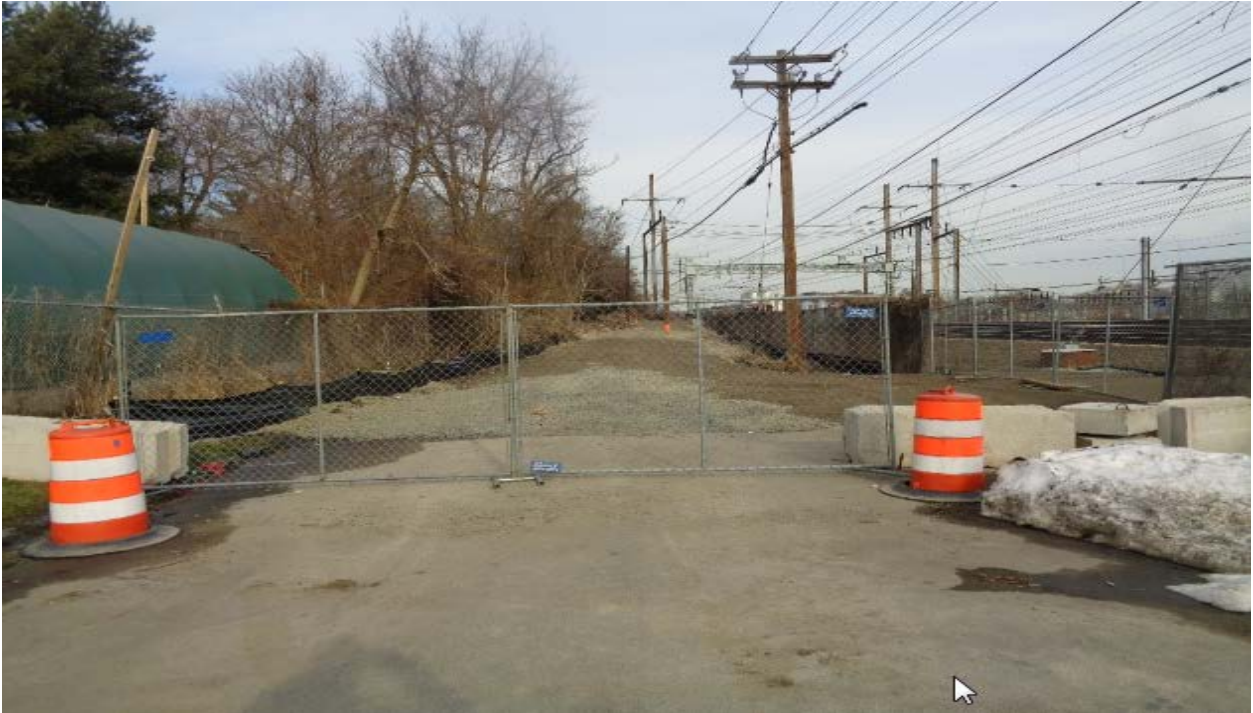
Construction entrance and access road to Structure(s) 821N, 822N, 823N and 824N
