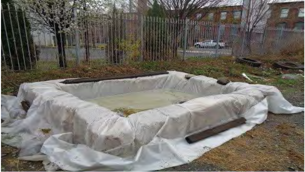
Washout area at Structure(s) 801S, 802S, 803S, 804S and 805S
