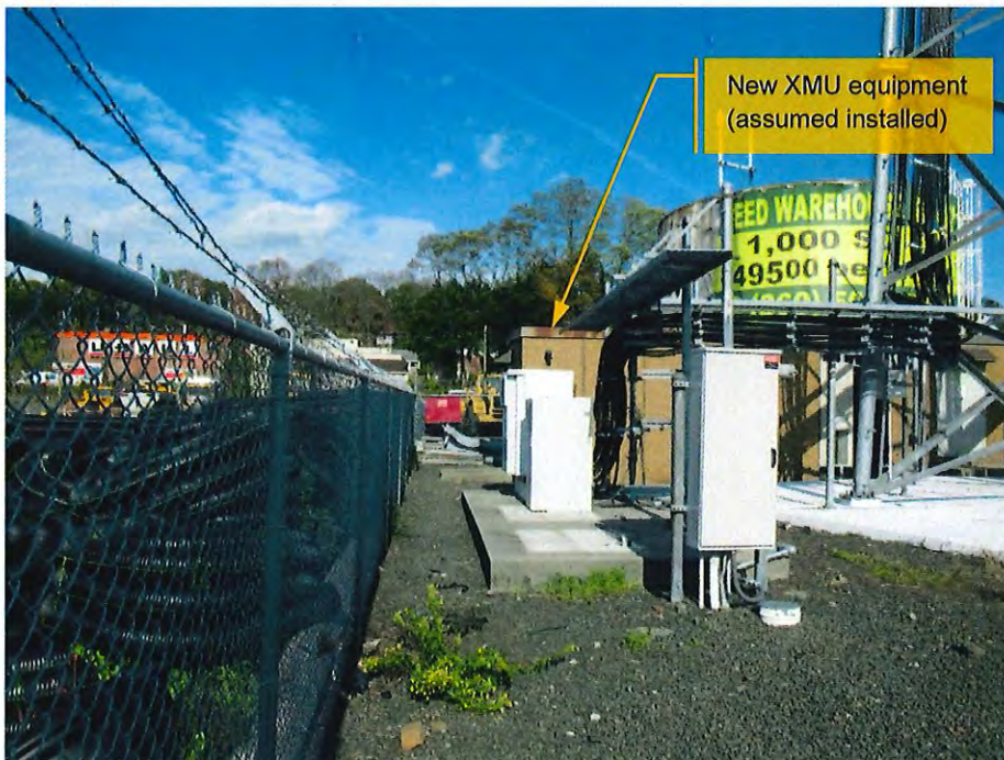
Photo 2 – Existing shelter with new XMU equipment assumed to be installed inside
