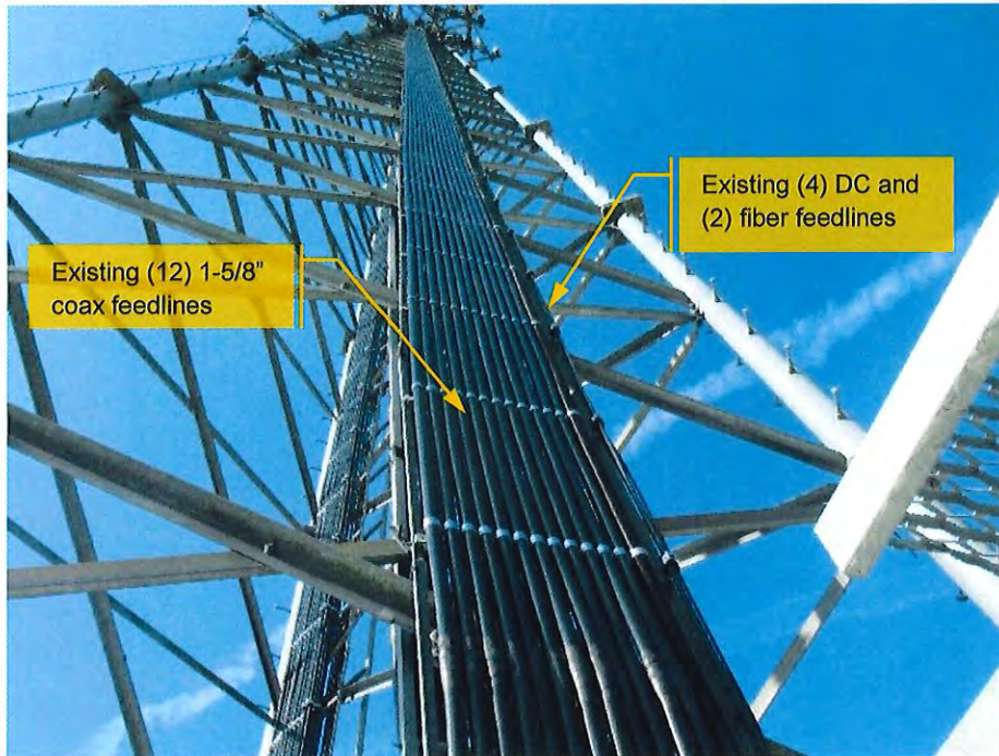
Photo 3 – Existing AT&T feedlines
