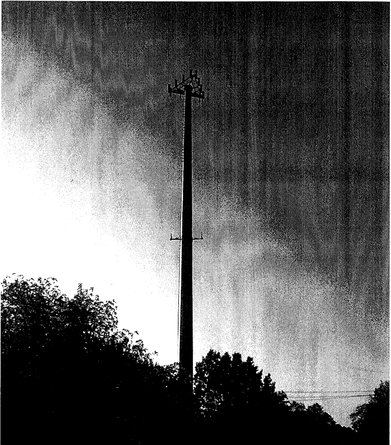
AT&T Wireless 1214 Farmington Ave Bristol 10/12/01
