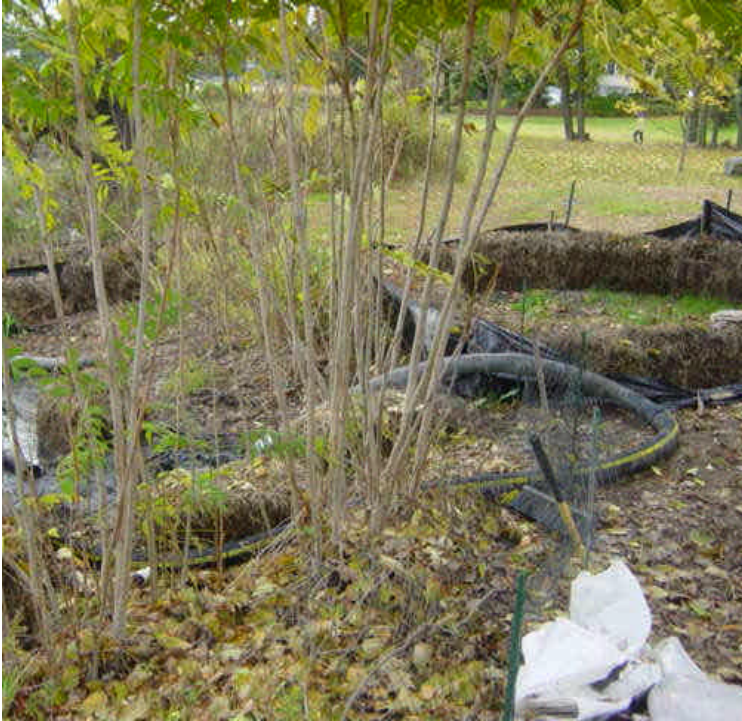
View of haybale filtering/dewatering area on the west side of the Saugatuck River. Pumped material is discharged into this area filter out the water; so that the remaining sediment and bentonite can be placed into the vac trucks for disposal.
