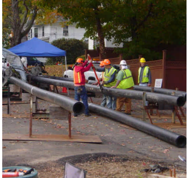
On the west side of the river, Lincoln St. has been closed off and conduit sections were being staged and fused together.
