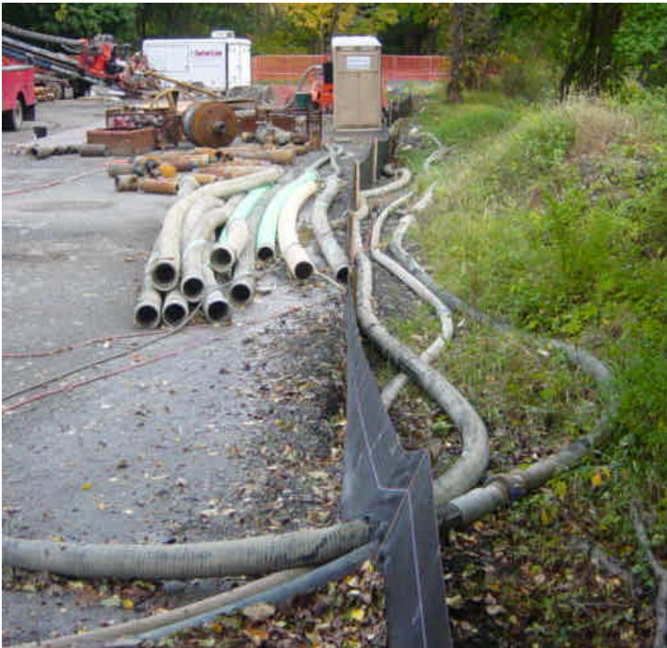
On the east side of the river, several hoses are being used in the HDD operation and are located outside of the contained, silt fenced limits of the staging area. Relocate hoses within the staging area to whenever feasible and construct forked (Y) stakes to prop hoses over the perimeter controls when necessary.
