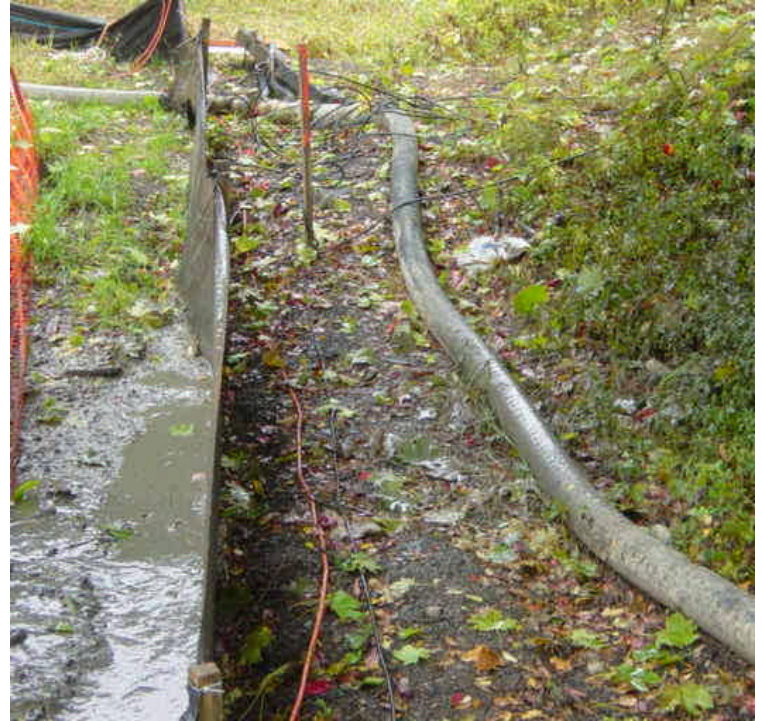
The perimeter silt fence appears to be adequately sized and positioned to contain the drilling slurry return and recycling pits on the east side of the river. However, some of the drilling fluid appears to have migrated out of the pit, against the fence. A small amount splashed beyond the controls.
