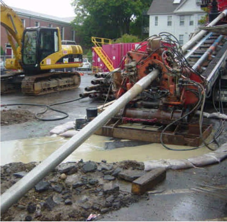
View of the drilling rig positioned in the staging area on the west side of the Saugatuck River. Drilling fluid is being properly contained.
