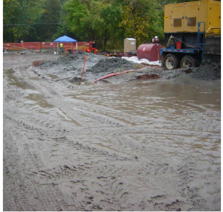
Staging area on the east side of the Saugatuck River was becoming very muddy as a result of the bentonite reclamation combined with the rain. The area was being adequately maintained and tracking was not an issue.
