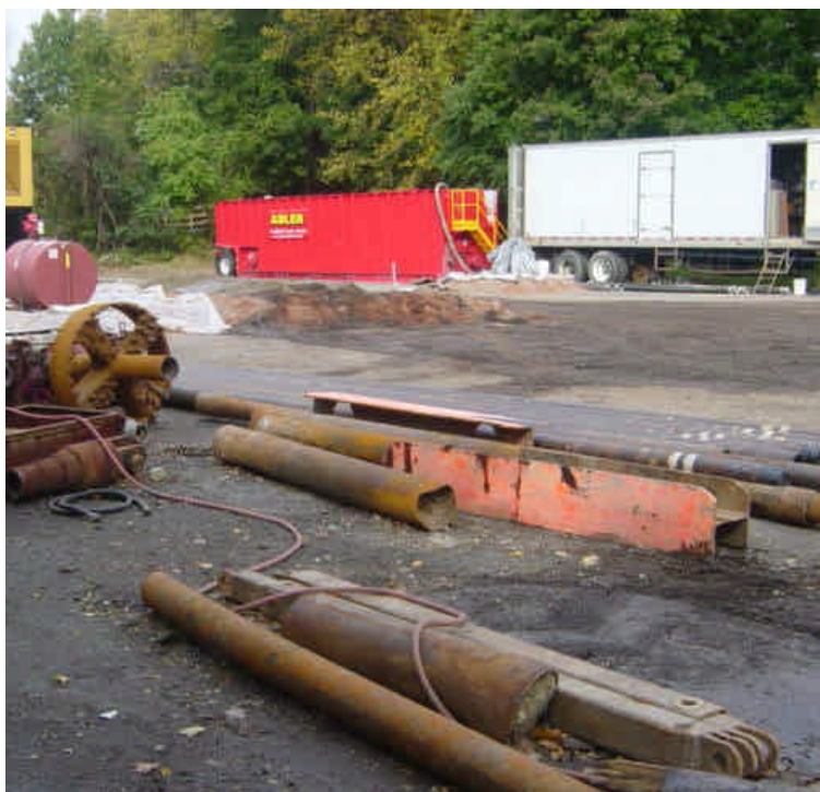
The staging area on the east side of the river remains fairly stable. Silt fence around the perimeter of the yard and around the drilling pit need attention.
