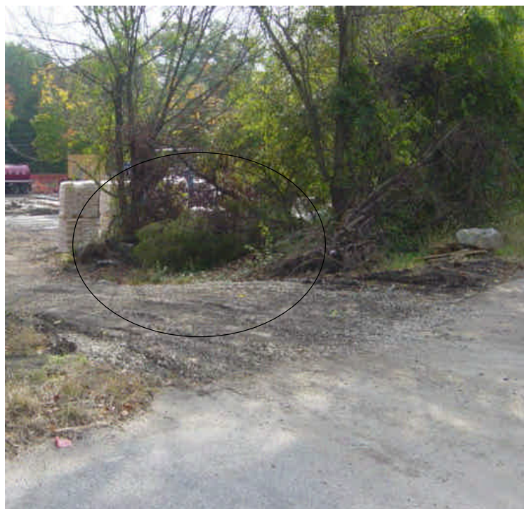
Tracking was previously observed at the entrance to the staging area on the east side of the river. The stone entrance has been refreshed but previously tracked sediment remains in the parking lot area.
