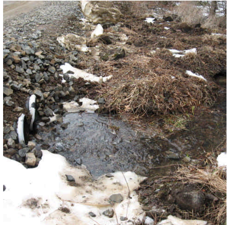
Cow Path Lane: Water flowing from the outlet pipe at the first crossing was free of sediment. 3/23/07
