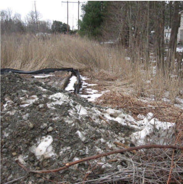
Hunting Hill Rd: Snow/sediment was piled on top of the silt fence and into the wetlands off the timber mats here. 3/23/07.
