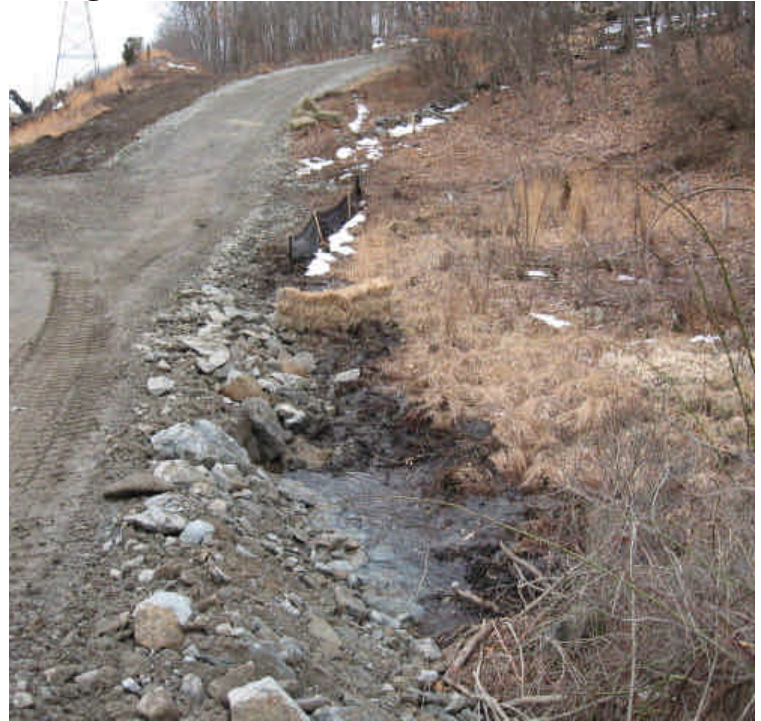
Check dams had been installed along the swale to a stream crossing. Controls were suggested on 3/19/07 and installed by 3/23/07. Continue to monitor and add controls as necessary.
