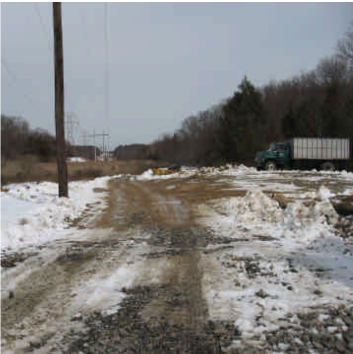
Cow Path Lane: A truck and sanitary facility were noted adjacent to wetland areas on either side of the ROW. Work space is limited here but attempt to provide storage away from wetlands. 3/19/07
