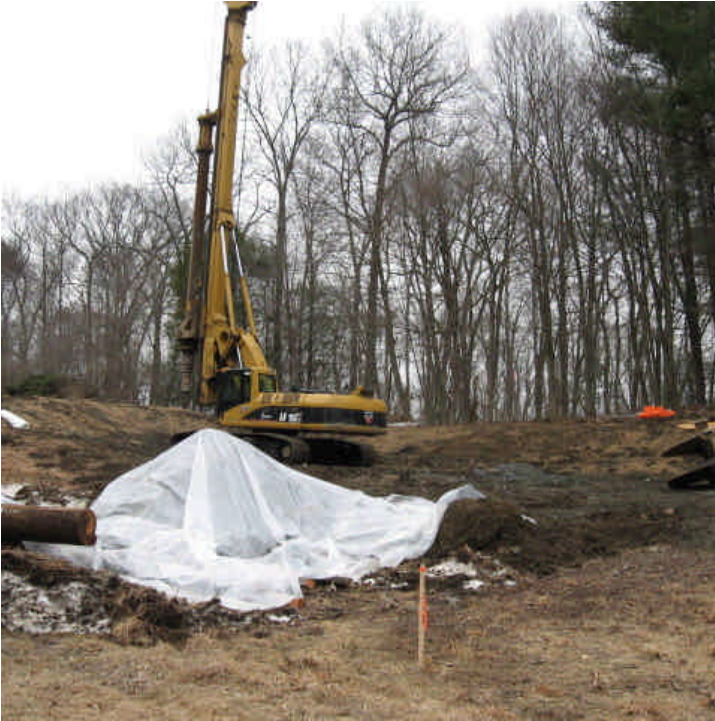
SCRWA, Morris to Dillon St (Woodbridge): Drilling has begun for structures #3950 A&B. 3/23/07.
