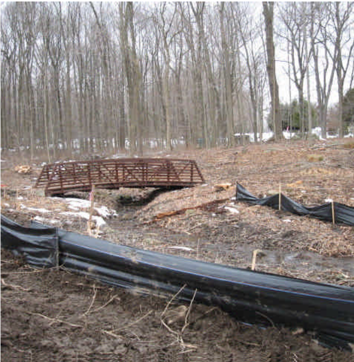
JCC Bypass (Woodbridge): Clearing activities appear to be complete in this area. Silt fence was in place along the stream. 3/23/07.
