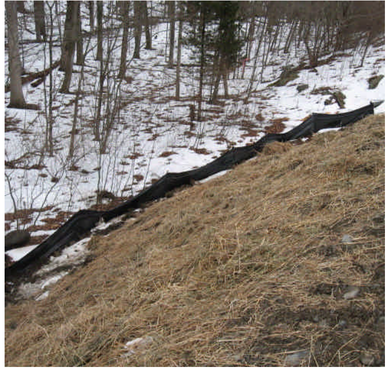
Cow Path Lane: Mulch was applied to the graded side slopes and silt fence remains in place by 3/23/07. The stream is located downgradient.
