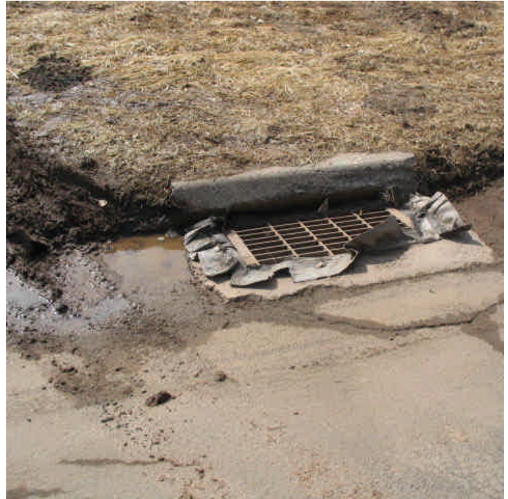
Old Lane Rd: The catch basin adjacent to the ROW access road is still receiving turbid runoff from the overhead ROW. There is no curb drop inlet protection here. 3/13/07.
