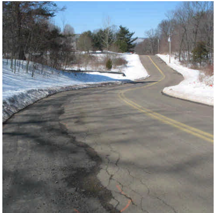
Old Lane Rd: No active work was noted within the roadway. Trenches have been backfilled and patched. 3/20/07.
