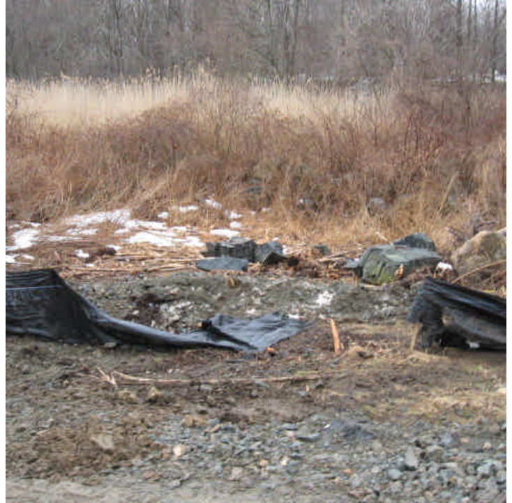
Whealers Farm Road: Silt fence remains damaged and is covered with sediment from plowing activities on 3/23/07. The small sediment pile should be carefully removed and place back on the work side of the fen
