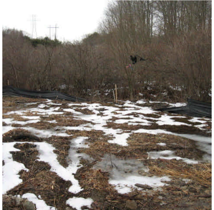
Route 121: It appears that the silt fence near the stockpile was repaired, but damaged by recent snow fall. 3/23/07.
