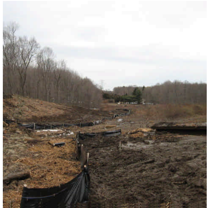
JCC Bypass: Silt fence was in place along the majority of the wetland area and was being extended at the time of inspection. 3/23/07
