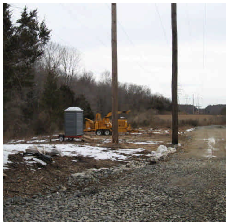
Cow Path Lane: The truck was no longer present on 3/23/07. An effort has been made to re-locate the sanitary facility, but due to limited work space and wetland configuration, options are limited.
