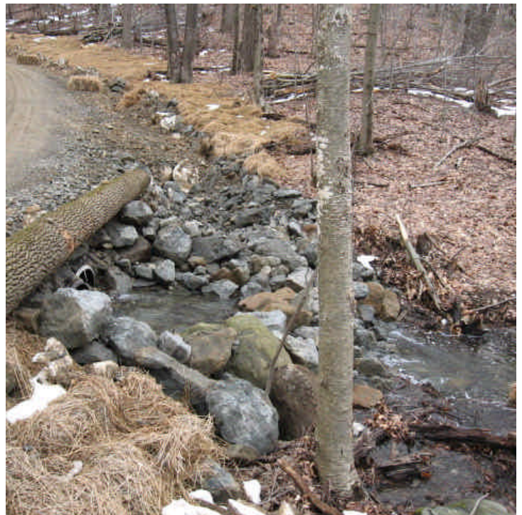
Cow Path Lane: View of the stream outlet on 3/23/07. A stone sediment trap was constructed at the culvert outlet and haybale check dams were installed downgradient.
