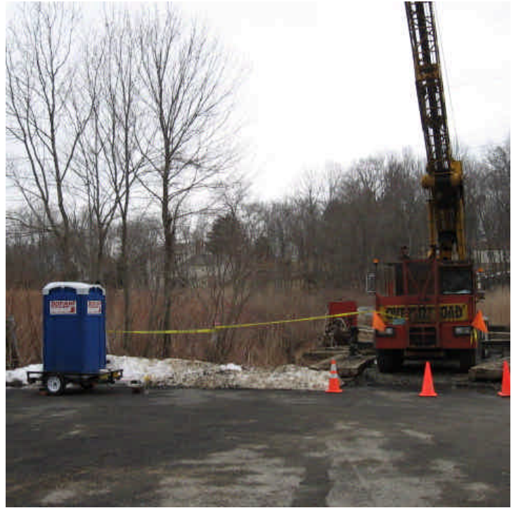
Hunting Hill Rd: Drilling equipment was being stored on a small upland area, adjacent to the wetland. The sanitary facility was removed from the wetland by 3/23/07. Workspace is limited here.
