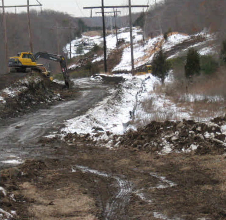
Cow Path Lane: Overall view of the activity within the ROW on 3/19/07. Major grading and soil movement was occurring to construct pads for structures.
