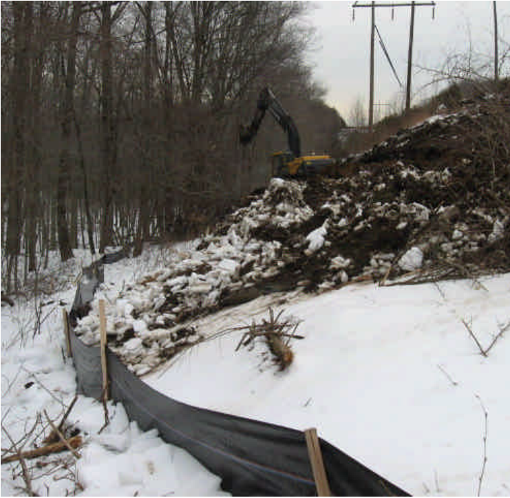
Cow Path Lane: Grading for pads resulted in some temp. soil stockpiling. Sediment and cleared snow were piled against the silt fence and had the potential to overwhelm the controls on 3/19/07.
