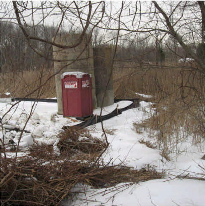
Hunting Hill Rd (Orange): A sanitary facility was noted within the wetland on the timber mats at the foundation drill site on 3/19/07.
