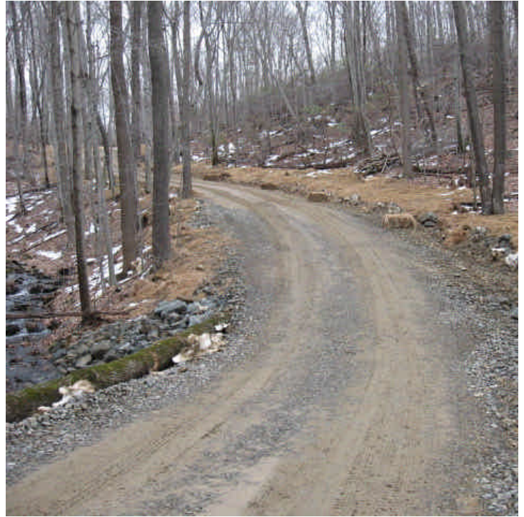
Cow Path Lane: View of the access road at the stream crossing on 3/23/07. Haybale check dams were in place along the access road and mulch had been applied to the disturbed slopes.
