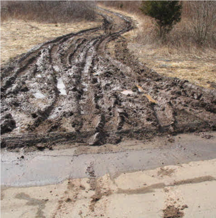
Old Lane Rd (Hamden): The entrance to the overhead ROW access road was very muddy this week. Sediment tracking was noted within the roadway. 3/13/07
