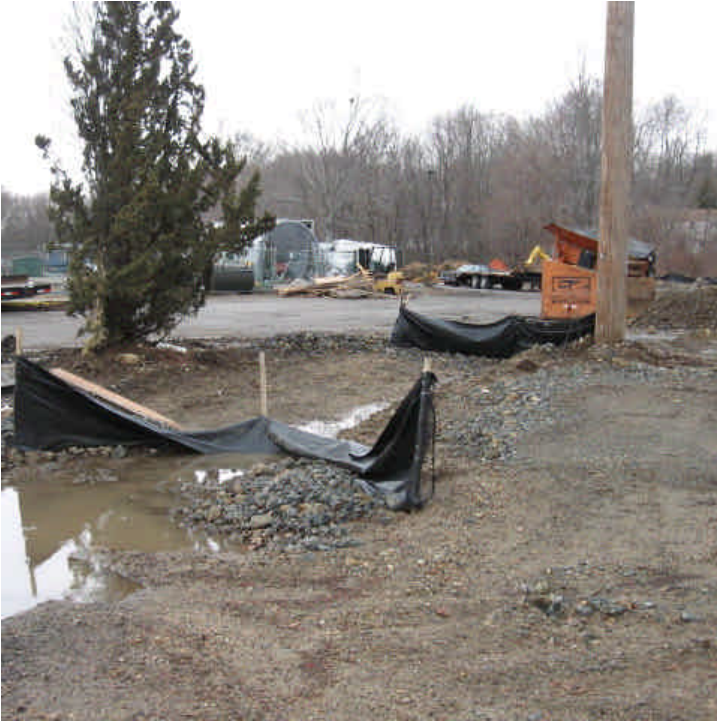
Route 121 (Milford): It appears the check dams were repaired but recent snow fall has damaged the silt fence again in this area. 3/23/07
