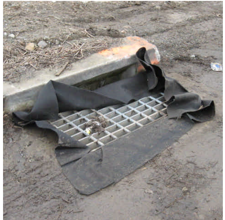
Silt saks were installed within the catch basins along Plains Road. Fabric was pulled over the curb inlets in some locations. 3/23/07.
