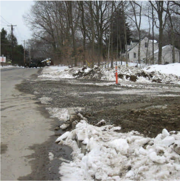
Shelland Street (new location) was very muddy at the time of inspection and some sediment tracking was noted on Plains Rd. 3/19/07.
