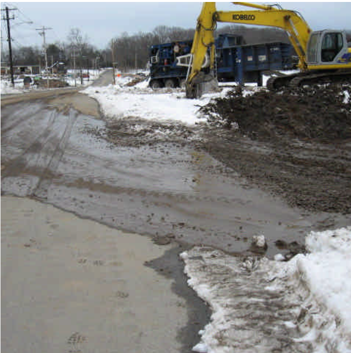
A significant amount of mud was being tracked into the roadway at the western construction entrance off Plains Road. 3/19/07.
