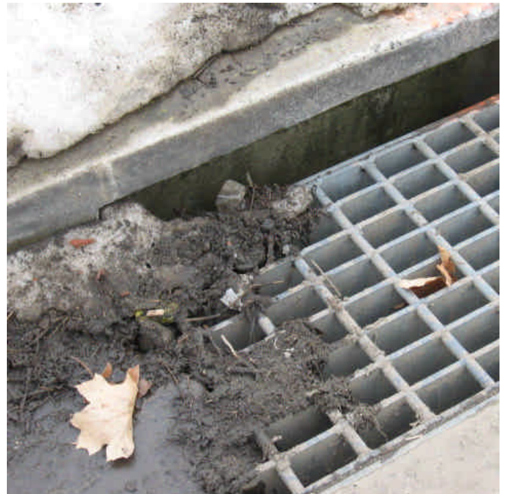
The catch basins along Plains Road were not protected with silt sacks or similar. Curb drop inlet protection was also not provided. 3/19/07.
