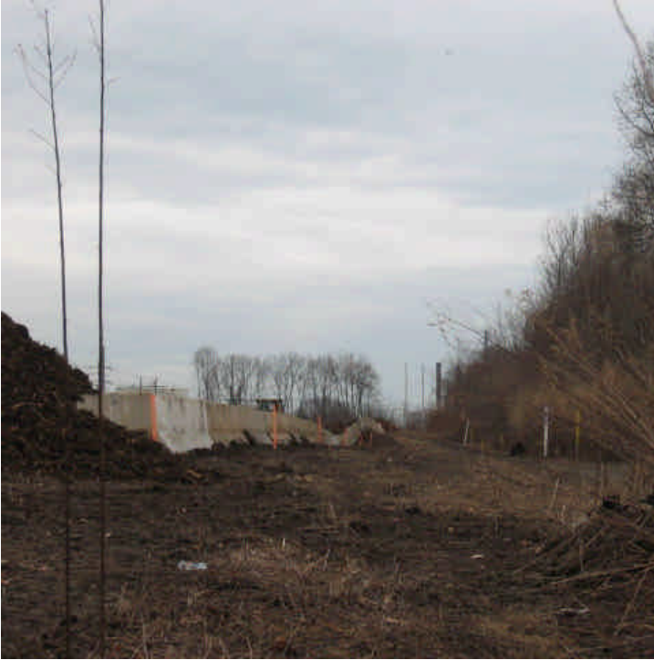
Jersey barriers were in place along the western boundary of the substation site. 3/23/07.
