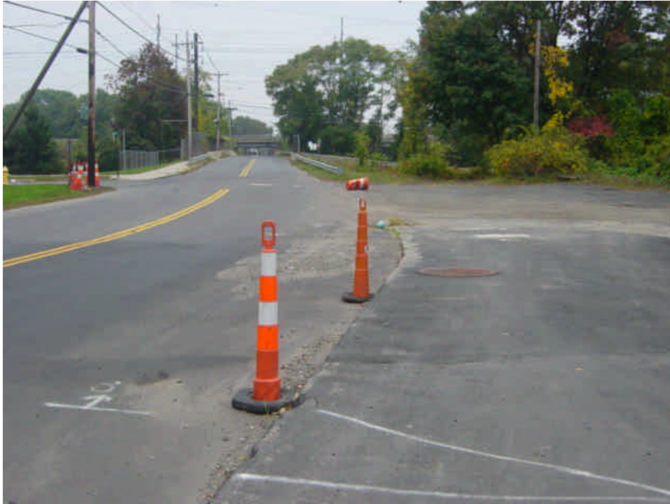
Staging area for the Metro North Railroad HDD along Naugatuck Ave remains unchanged from the previous week. Sediment and sand remains in and around the catch basin. The catch basin needs to be cleaned out.
