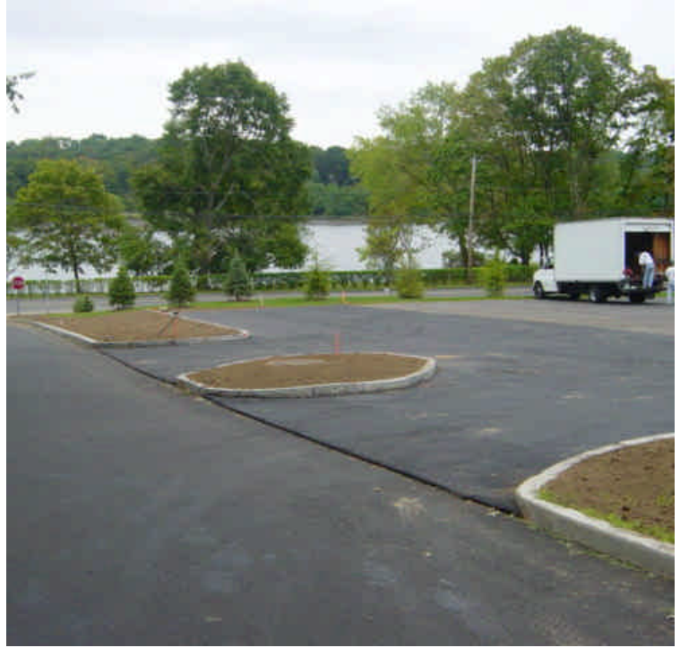
Parking lot near sta. #234 has been repaved and the island areas appear to have been seeded. Provide mulch to prevent exposure to erosion.
