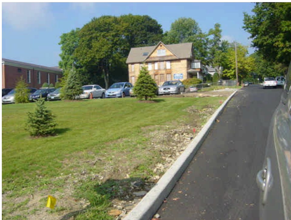
On the west side of the Saugatuck River, curbing has been reset along Lincoln Street. Continue to stabilize the soil located immediately adjacent with grass cover.
