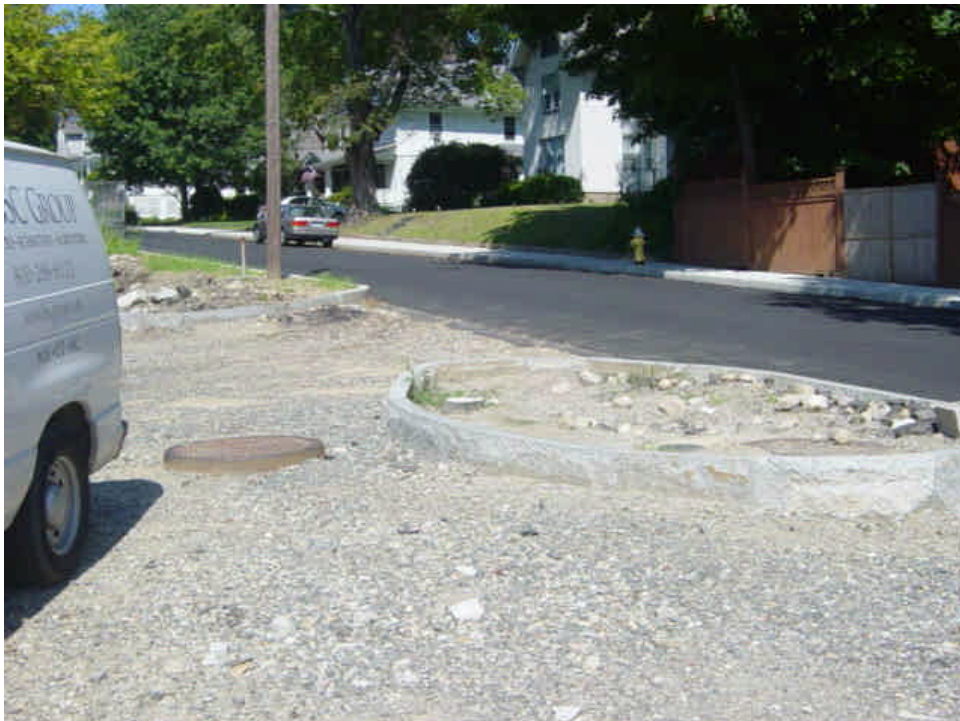
On the west side of the Saugatuck River stone curbing has been set and soil has been spread in some areas. Final surfacing is needed here as soon as possible.
