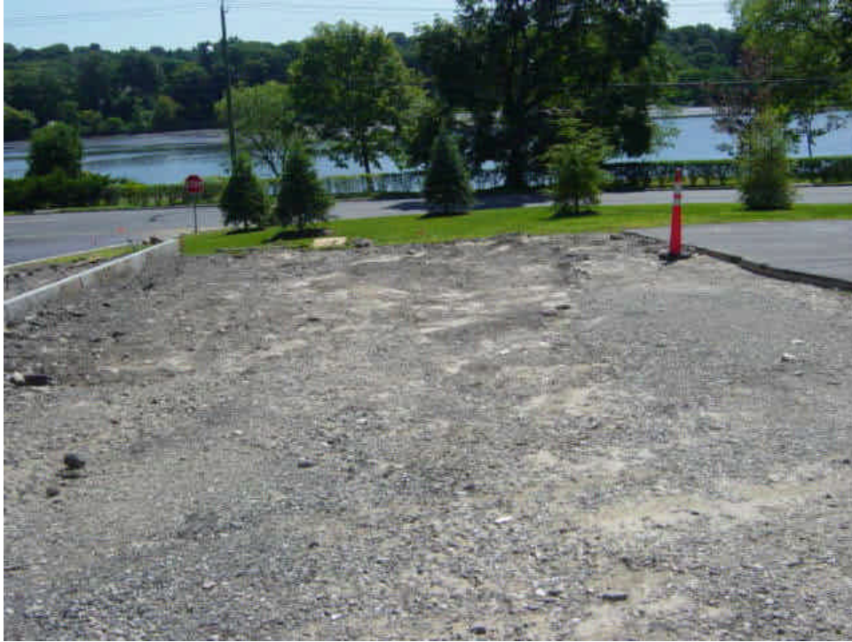
On the west side of the Saugatuck River, portions of the work area have re-vegetated. The adjacent area is still waiting to be paved (since 3/20) with the potential for run-off.
