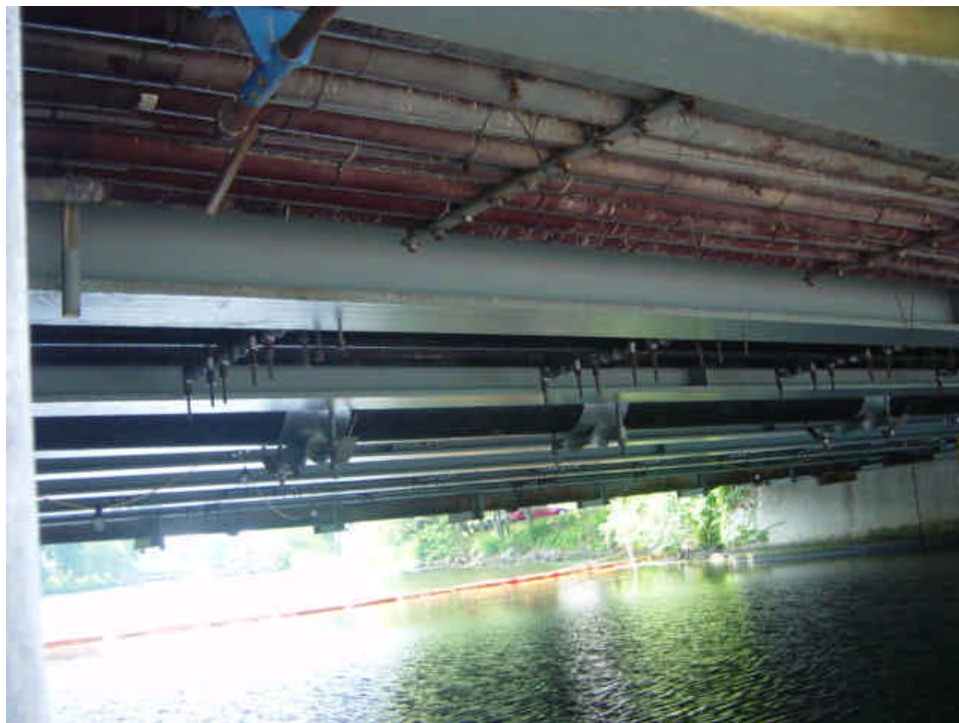
Conduit has been attached to the bridge over the Mill River (Southport Harbor).
