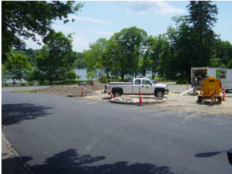
On the west side of the Saugatuck River, the staging area is still waiting to be paved. Stone curbing has been set and soil has been stockpiled in these areas. Minor tracking was observed on Lincoln St. New River Electric was on-site.
