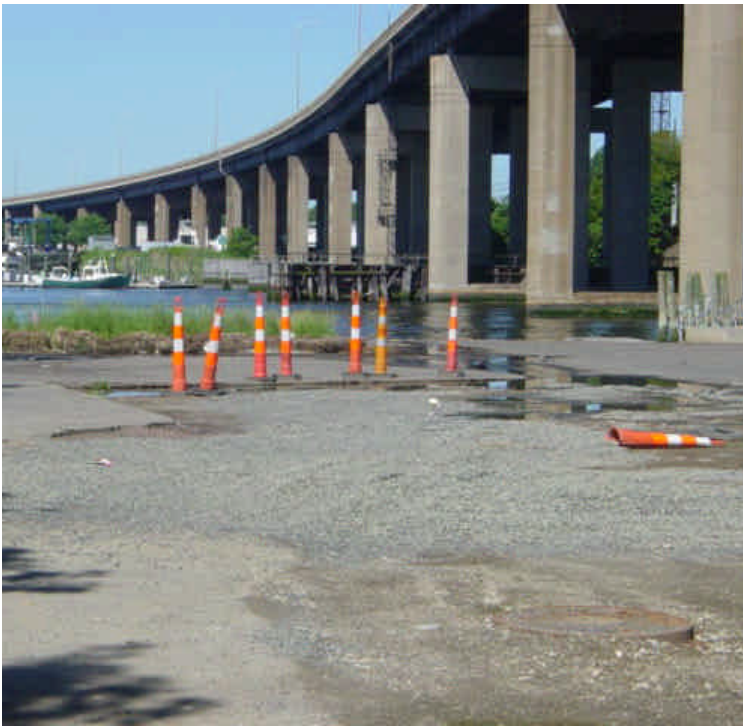
Hay bales remain along the east bank of the Housatonic River, and the area is ready to be paved. The surface should be stabilized as soon as possible as this area appears to have the potential to be inundated.
