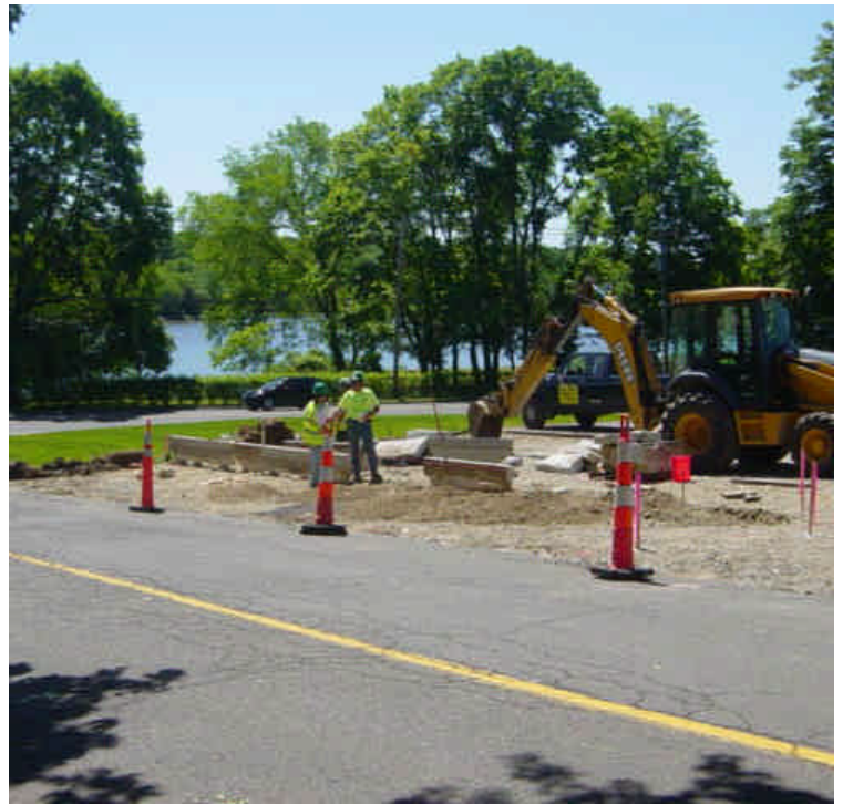
On the west side of the Saugatuck River, the portions of the work area that were restored are vegetated. The adjacent area is still waiting to be paved. Stone curbing was being set and electrical contractors were on site pulling cable.
