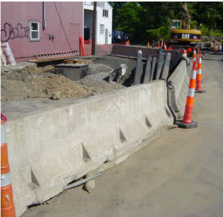
Tie-in work for one of the two circuits has been completed on the north side of the Metro North R.R. Crossing. Accumulated sediment has been swept from along the edge of the roadway. A filter boom has been installed along the edge of the barrier curb to filter runoff.
