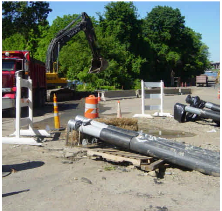
The staging area on the south side of the Metro North R.R. Crossing has been demobilized and the perimeter controls have been removed. Hay bales remain in one location near the drill pit where a minor amount of groundwater was observed seeping under the barrier. The runoff was generally clean and was flowing back towards the adjacent trench work.
