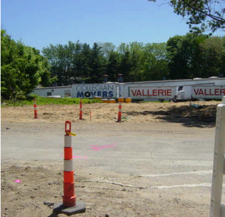
The area near the access drive to the boat ramp where the drilling rig was previously located has been partially restored. Hay mulch has been spread to stabilize the area.
