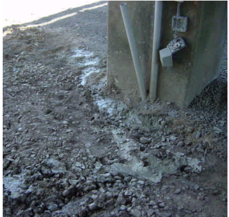
A minor amount of residual drill slurry was observed near the base of bridge foundation.
