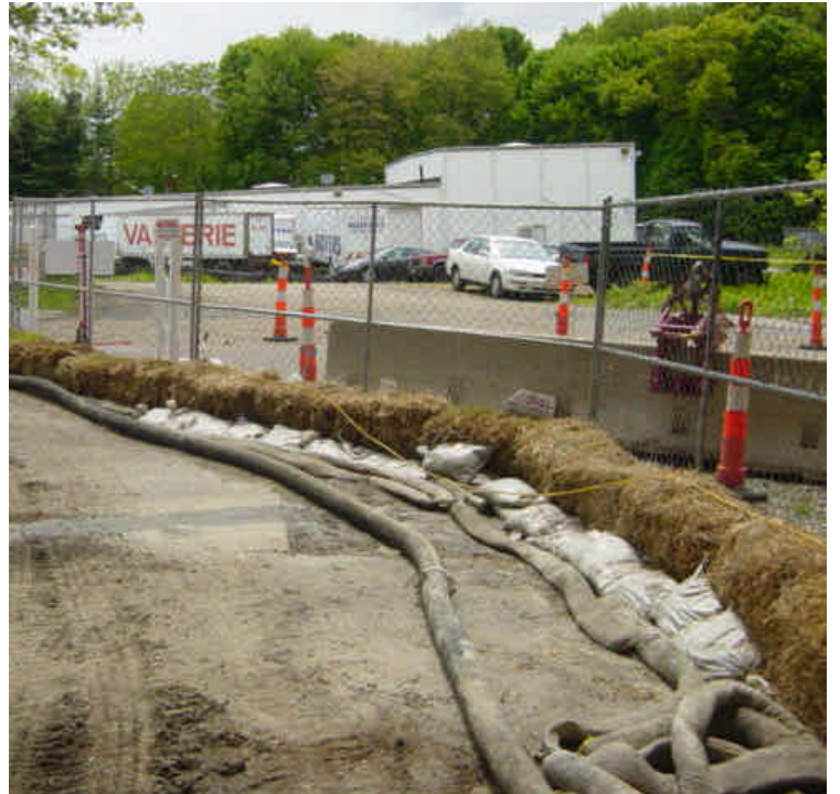
Perimeter barrier controls remain in place around the staging area at the Metro North Railroad Crossing in Milford. Continue to adjust as necessary.
