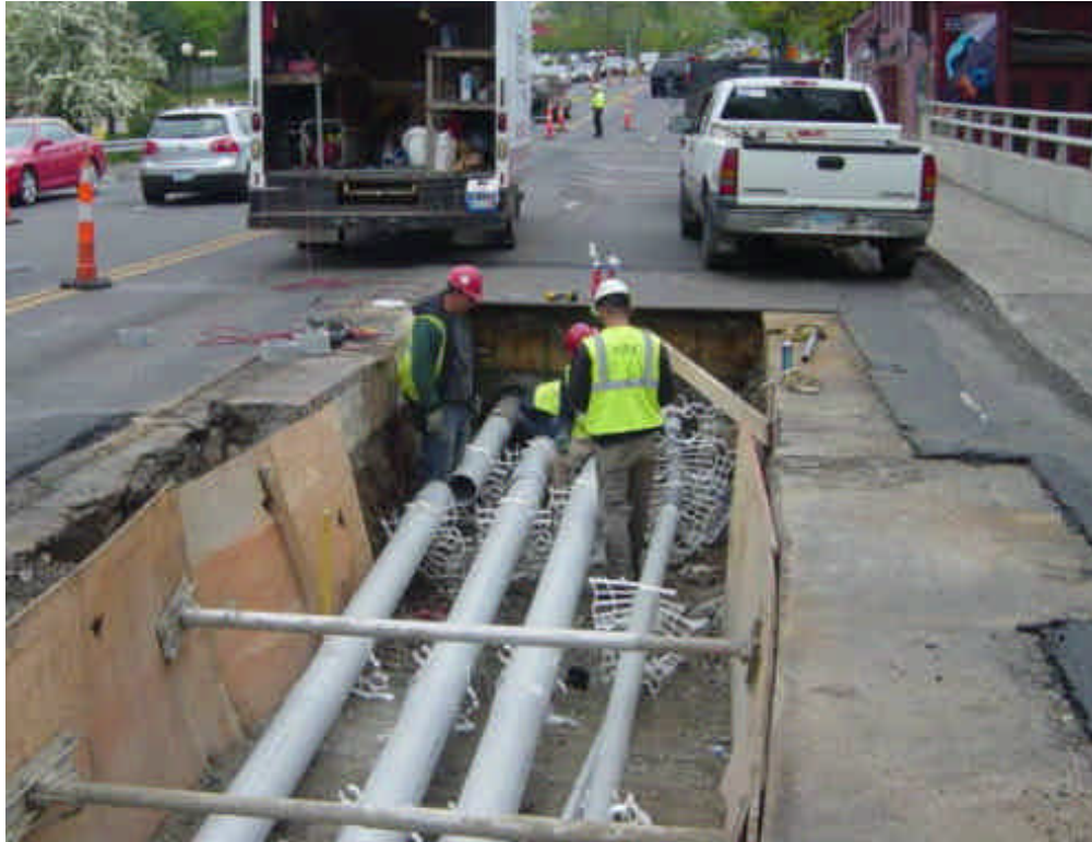
Electrical contractor was installing conduit banks at sta. #441, connecting/tying-in to the conduit sleeves attached to the bridge deck at Sasco Creek.
