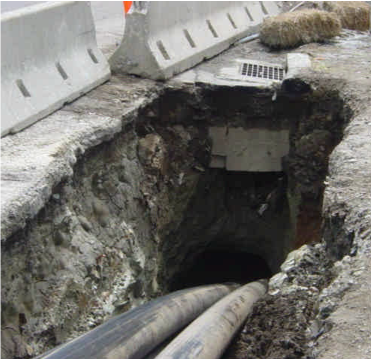
Conduit was being pulled through the second boring at the Metro North Railroad Crossing in Milford. Catch basin will still need attention.
