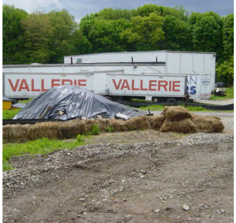
The soil stockpile located adjacent to the staging area near the Metro North Railroad in Milford has been covered with a tarp for further containment.
