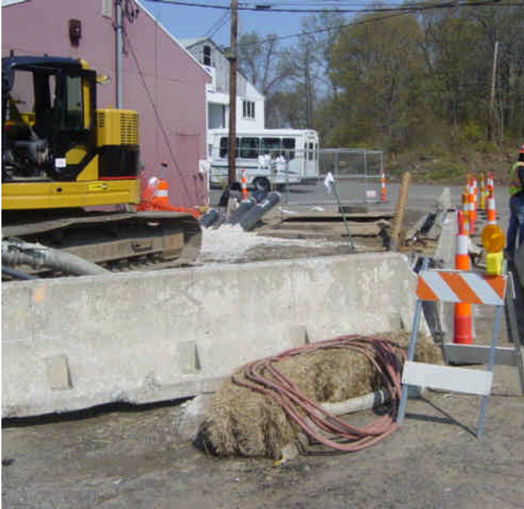
HDD work continues along Naugatuck Ave. The adjacent catch basin has been protected with hay bales and filter booms.
