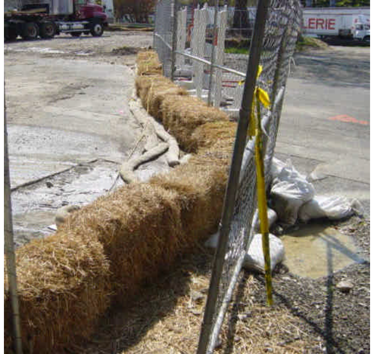
Sediment laden runoff/ slurry material was observed seeping under the hay bale barrier and beyond the fenced perimeter of the work zone in one location. Adequately control this material.
