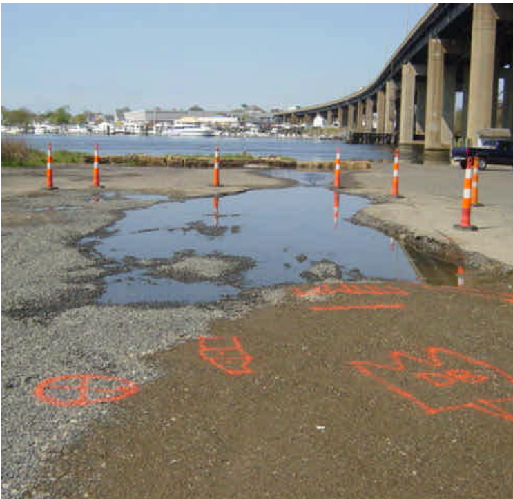
HDD work at the Housatonic River is complete. The drill pits have been backfilled and the west side has been paved. The conduits on the east side were inadvertently crossed during tie-in work and need to be partially excavated and corrected.
