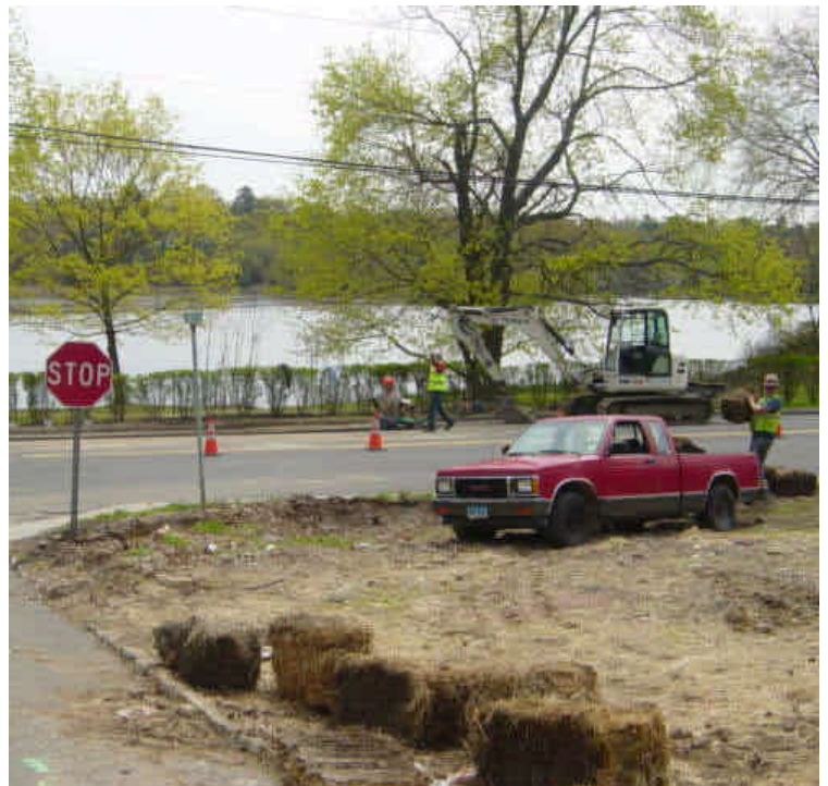
Shrubs previously removed the west side of the river near sta. #235+75 (not per the D&M) have been replaced. Hay bales were also being removed from along Riverside Dr. Continue to monitor until vegetative cover has establish in previously exposed areas.
