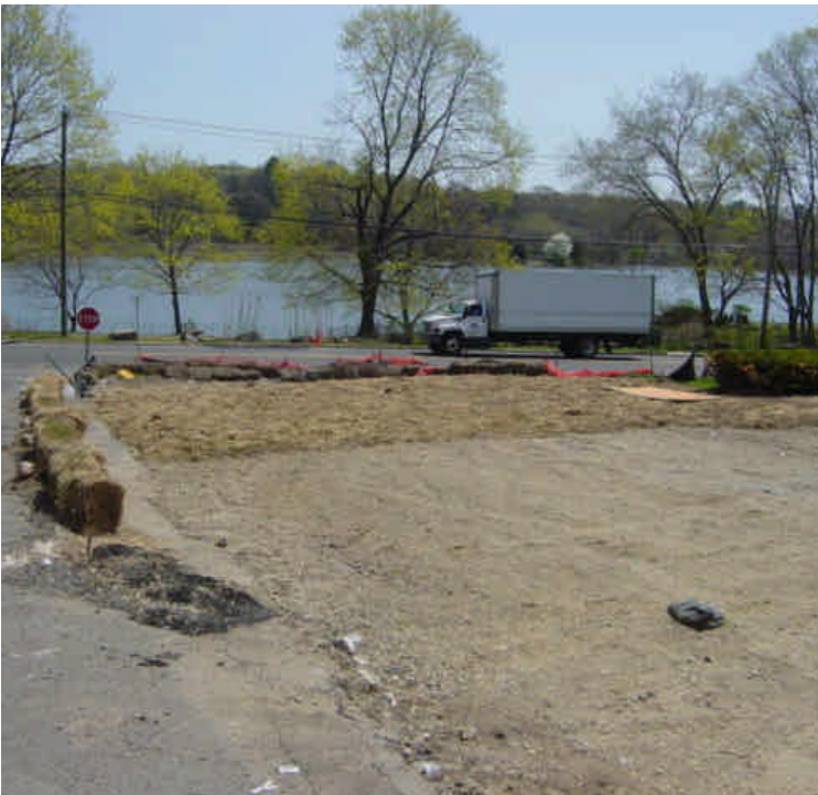
The area near sta. #231-234 has been prepared for paving for several weeks. Seed and mulch were previously spread over the areas of exposed soil that are not slated for paving.
