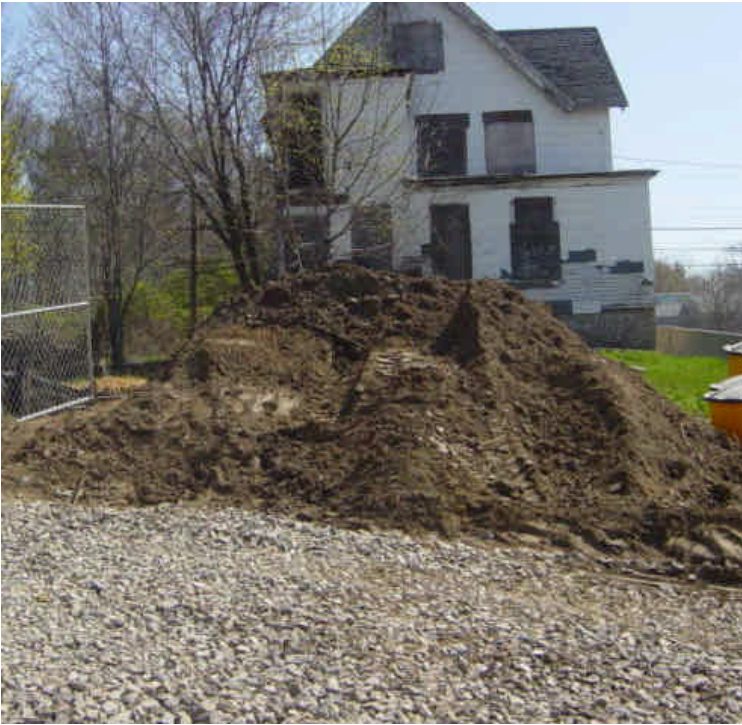
A new temporary access drive has been constructed at the Metro North Railroad crossing in Milford. Stockpiled soil is being stored outside of the controlled area and lacks adequate containment.
