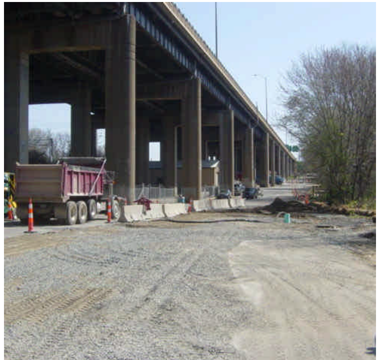
HDD vault tie-in work has been completed on the east side of the Housatonic River and the area has been backfilled in preparation for paving.
