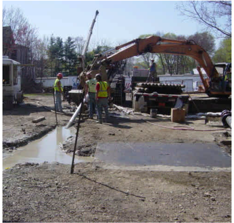
HDD work continues at the Metro North Railroad crossing in Milford. The drilling pit appears to be appropriately sized.
