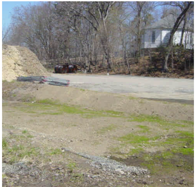
Work is complete on the east side of the Saugatuck River near sta #251. The area is partially restored. Wood chips and chain link fencing remain stockpiled in the staging area. A dirt berm was recently re-graded and grass cover is beginning to grow. Controls may be needed until the area is stable.
