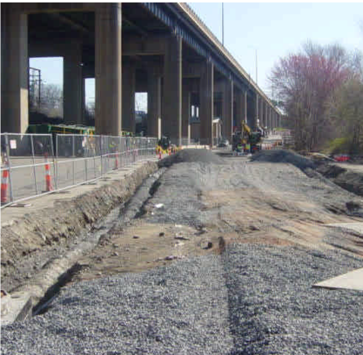
On the east side of the Housatonic River, vault tie-in work is nearing completion. Hand holes were being installed before the area is backfilled completely.
