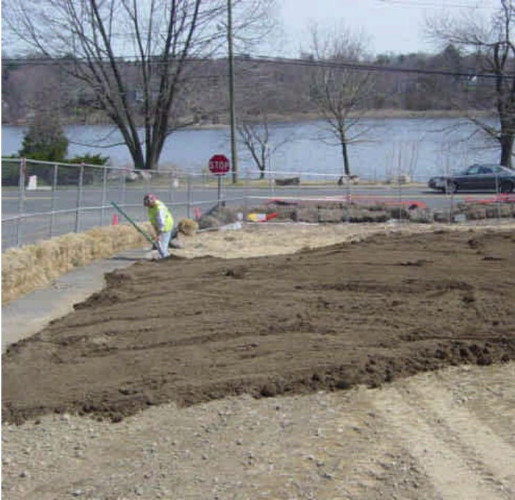
On the west side of the Saugatuck River near sta. #234, topsoil was being spread and the area was being seeded.
