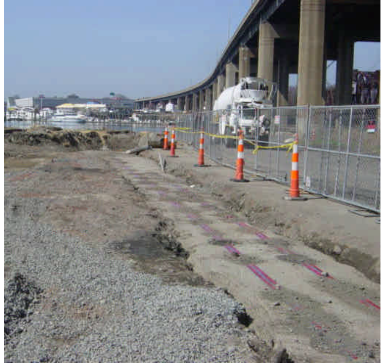
HDD work has been tied-in to the vault near sta. #1015 and the area has been partially backfilled. Final restoration or paving is still scheduled.
