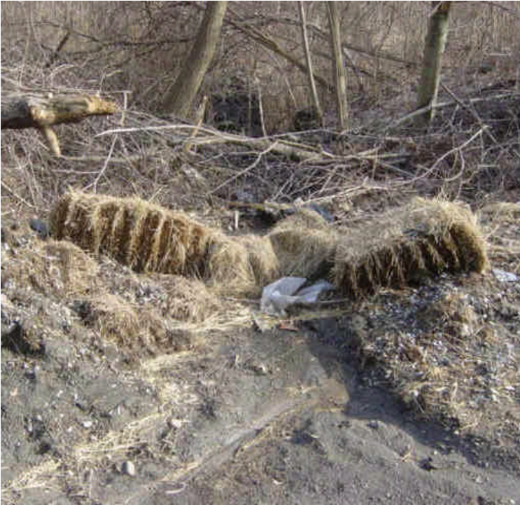
A small channel has eroded near the west side of the staging area on the east side of the Housatonic River. Haybales are in place and are containing most of the sediment, but a minor amount has migrated beyond the haybale barrier.
