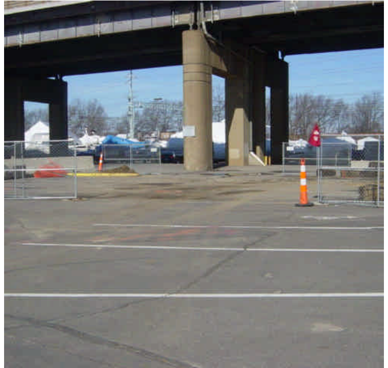
Staging area on the west side of the Housatonic River remains active as crews are working to tie-in the conduits to the existing vault. A minor amount of remnant sediment has accumulated and been tracked over the paved area.
