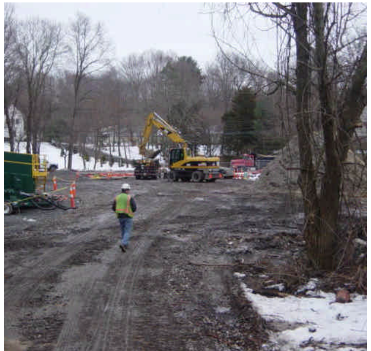
Staging area on the east side of the Saugatuck River was partially restored but is now being utilized by Seg. 4B contractors for the vault installation. Final restoration efforts will need to be coordinated between the contractors.
