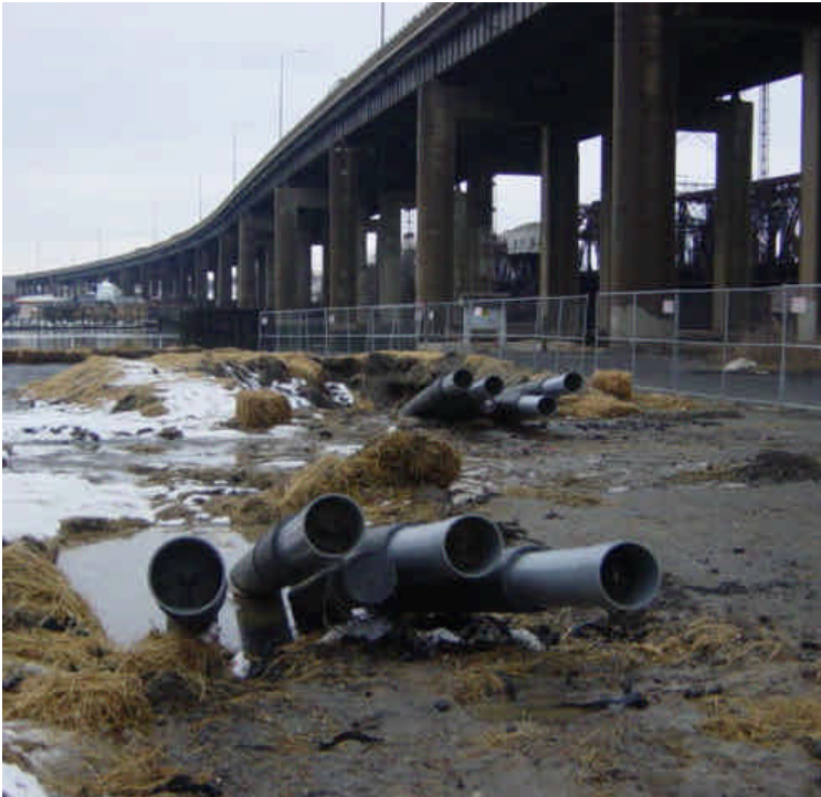
On the east side of the Housatonic River the dirt berms remain between the drill pits (conduits) and the river.
