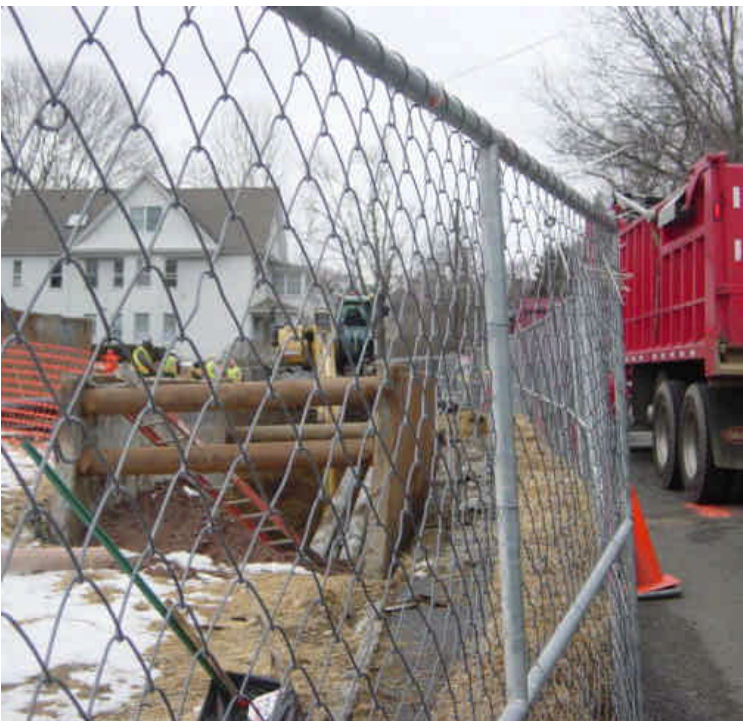
On the west side of the Saugatuck River, the HDD has been Completed and crews are now working on vaults and tie-ins.
