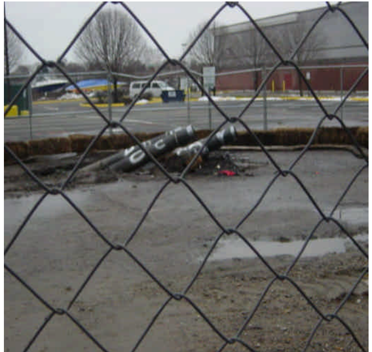
On the west side of the Housatonic River, the drilling pits have been backfilled, with only the conduits left exposed.
