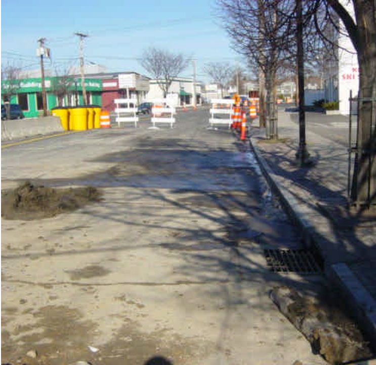
The drilling rig and bentonite reclamation machine have been removed from the temporary work zone at Ash Creek. A minor amount of sediment and debris remain throughout the work area. Hay bales protecting the catch basins have been removed.
