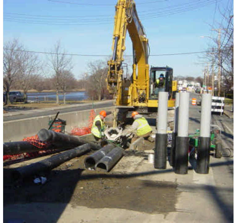
Crews at Ash Creek are fusing the final sections of conduit and preparing to cap the ends and temporarily backfill the drilling pit.
