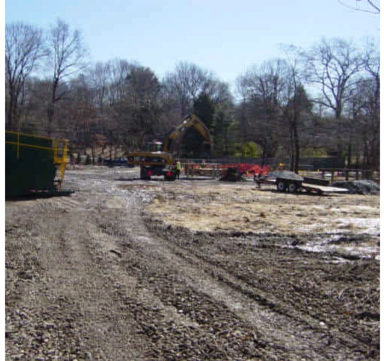
The staging area on the east side of the Saugatuck River has been partially restored. Additional restoration efforts are still required in some areas.
