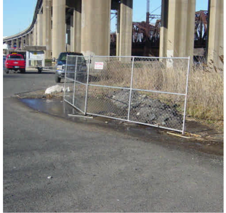
On the east side of the Housatonic River just adjacent to the work area, a small section of pavement had collapsed due to drilling activities. The area remains fenced.
