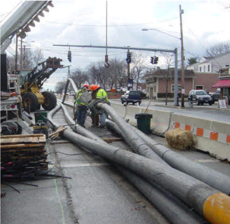
Crews at Ash Creek are fusing the final sections of conduit and preparing to pull the conduit through the boring.
