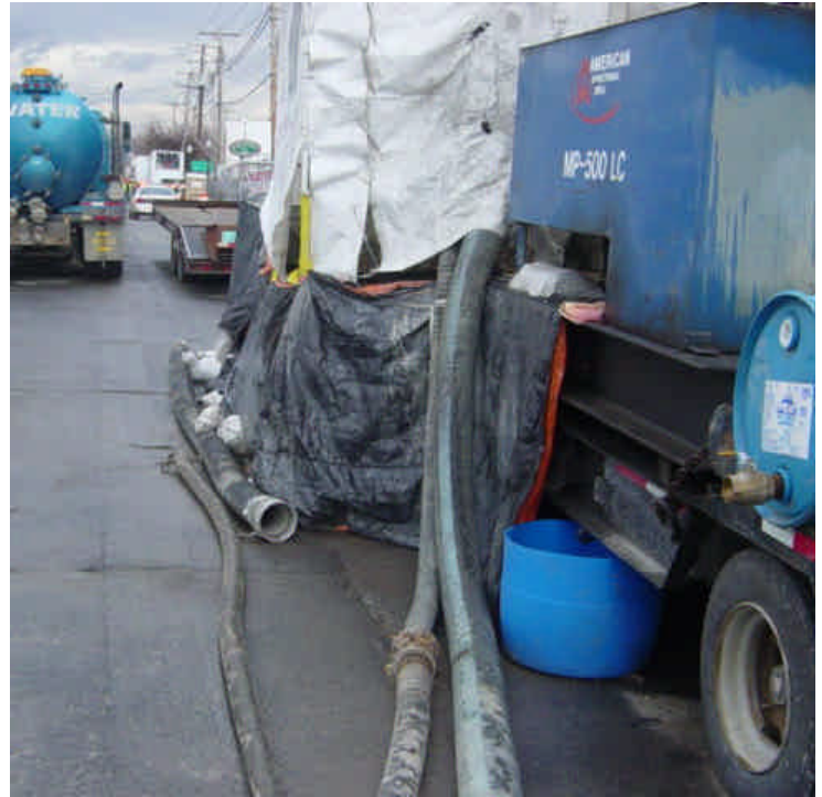
At Ash Creek, a large bucket has been placed under a piece of equipment to contain any leaking fluids.
