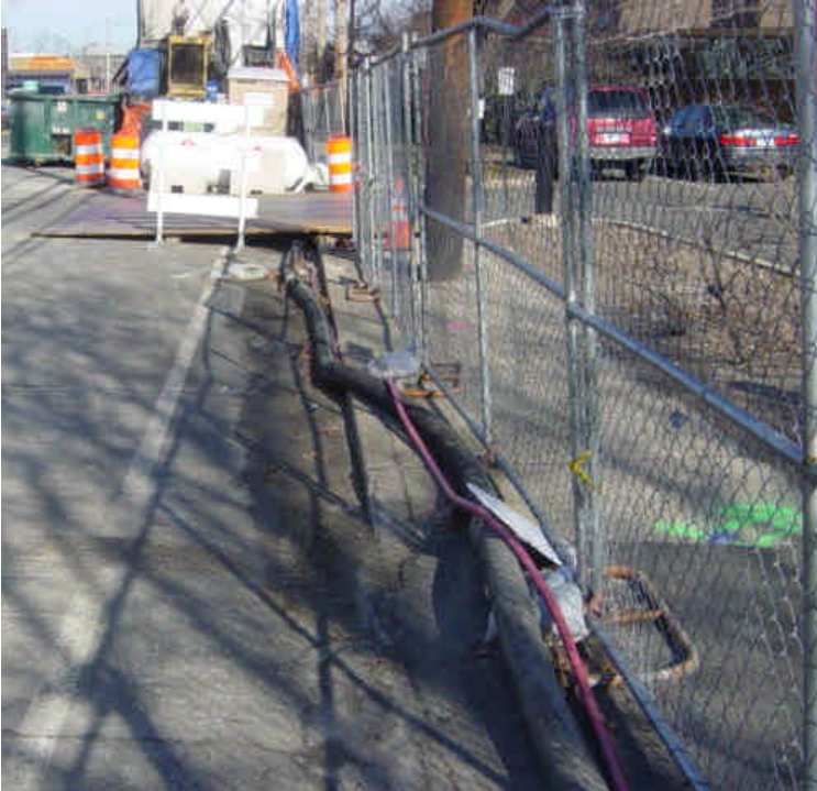
Sediment has accumulated along the curb on Post Road near Ash Creek. Continue to sweep work area to reduce tracking and unnecessary impacts.
