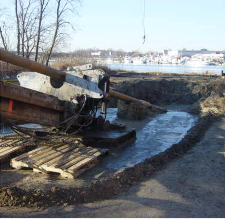
On the east side of the Housatonic River the drilling pit is adequately contained with a sand berm. Hay mulch also remains on portions of the containment berm for stabilization.
