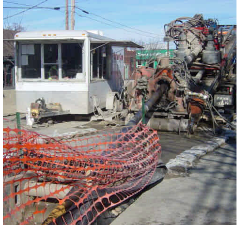
On the east side of Ash Creek, drilling continues. The drilling pit is adequately contained with sand bags. Some of the bags are deteriorating as a result of the changing temperatures and may need to be replaced.
