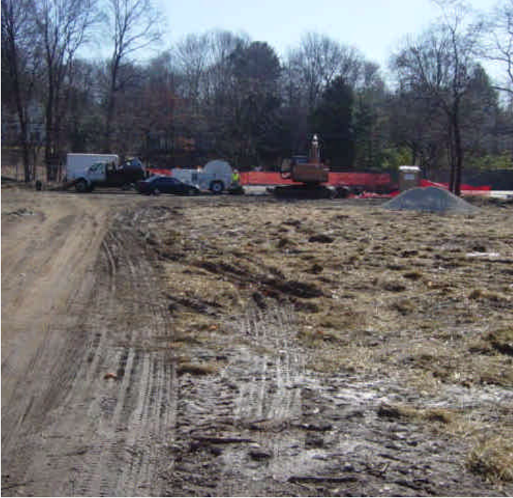
On the east side of the Saugatuck River, most of the drilling equipment has been removed from the staging area. Some minor ruts were noted off the edge of the access drive.
