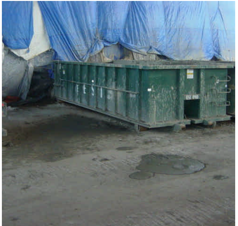
Mud and slurry material were observed on the paved surface near the bentonite reclamation machine.
