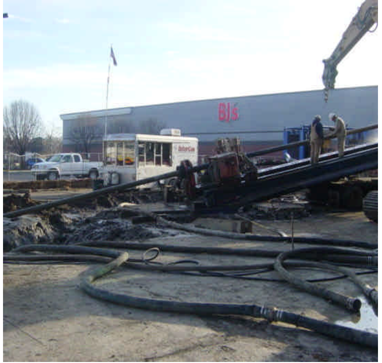
On the west side of the Housatonic River, a minor amount of slurry/mud was noted on portions of the paved surfaces in several areas throughout the staging yard.
