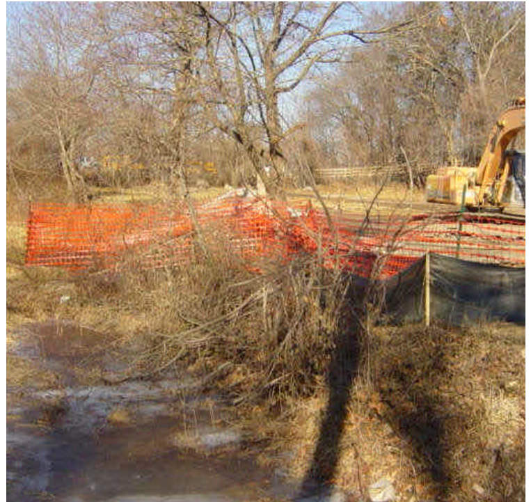
On the east side of the Saugatuck River, two small holes have formed between the drilling pit and the access drive. The area will need to be properly cleaned, stabilized, and backfilled.
