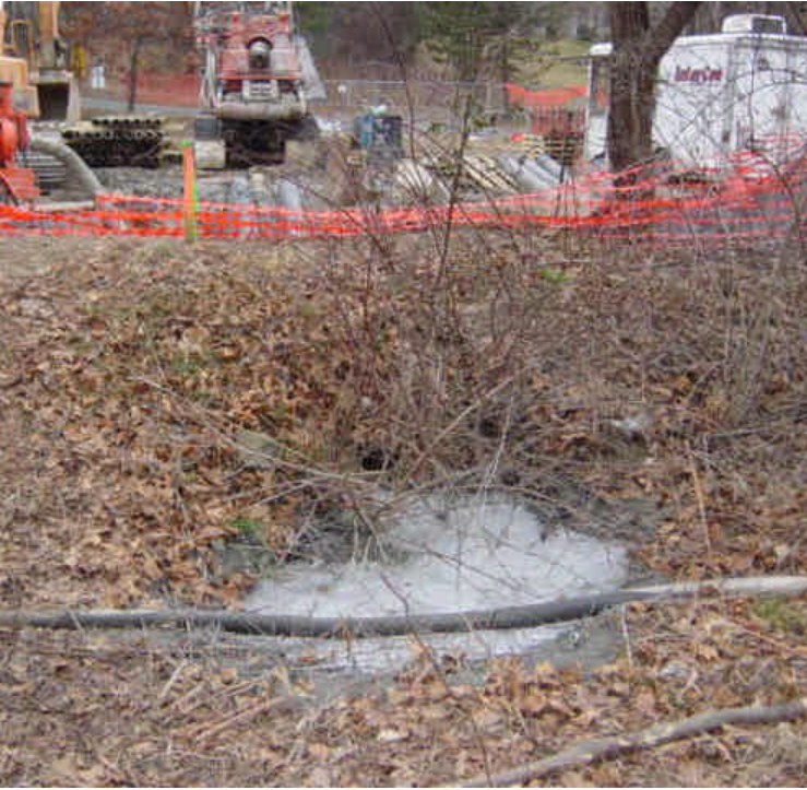
On the east side of the Saugatuck River two minor frac outs were observed on land between the access drive and drilling pit. The slurry material should be contained, and properly removed.
