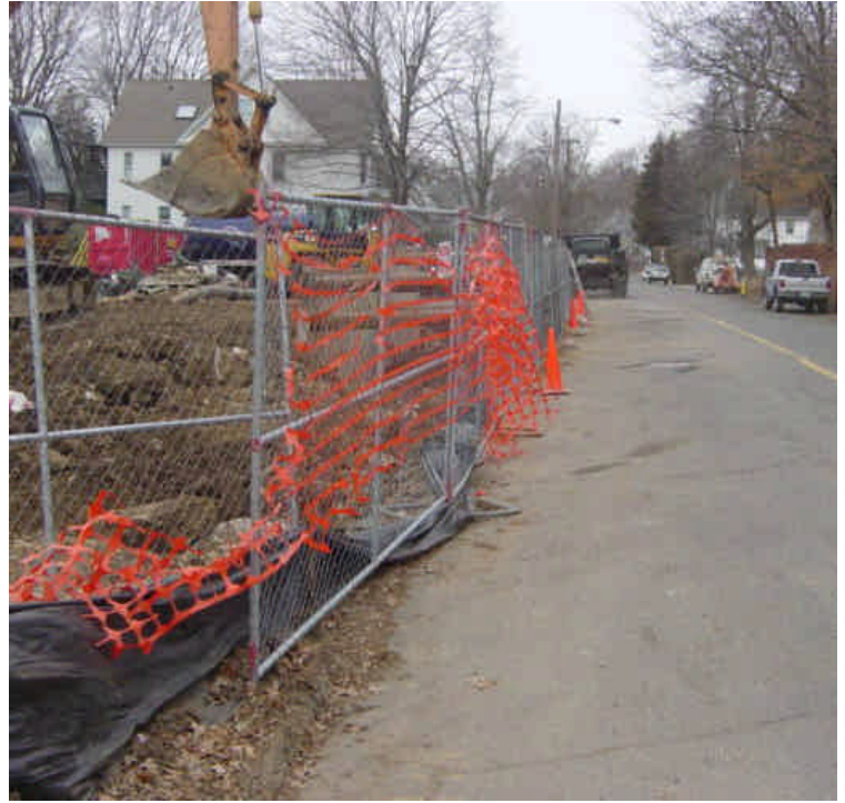
On the west side of the Saugatuck River, the silt fence along Lincoln Street needs repair.
