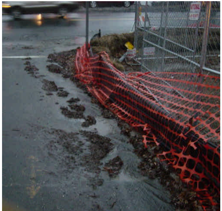
On the west side of the Saugatuck River, runoff was carrying sediment downgradient into a protected catch basin. Attention is needed to keep sediment off the roadway.
