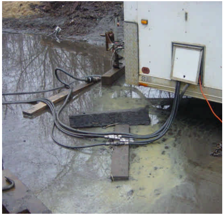
On the east side of the Housatonic River, sediment remains on the paved area. The sediment should be removed prior to work resuming in this area to reduce potential tracking or unanticipated impacts.
