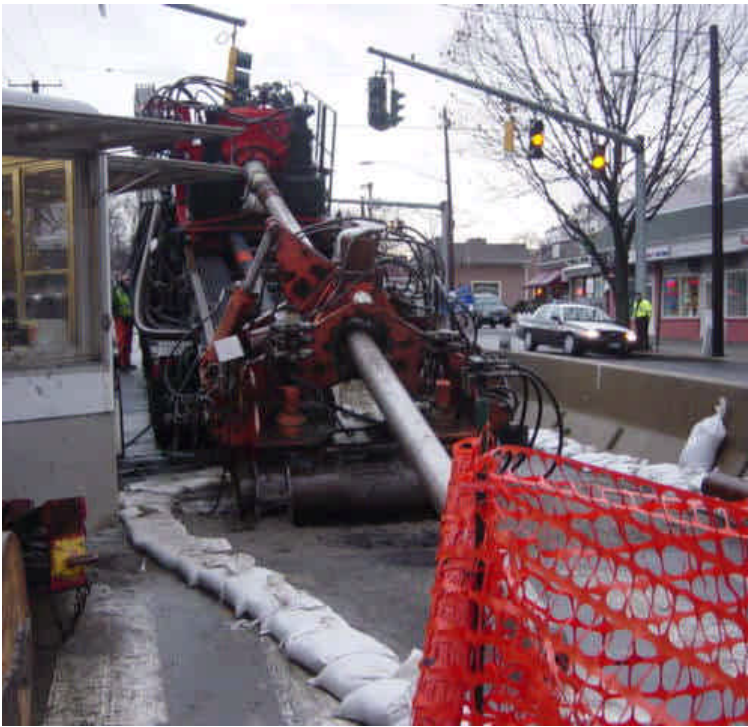
On the west side of Ash Creek, work has resumed following the break. The drill rig remained in place while work was temporarily inactive due to mechanical problems.
