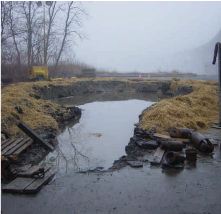
On the east side of the Housatonic River, the earthen berm and hay bales around the drill pit appeared to be functioning well. The berm was recently mulched.
