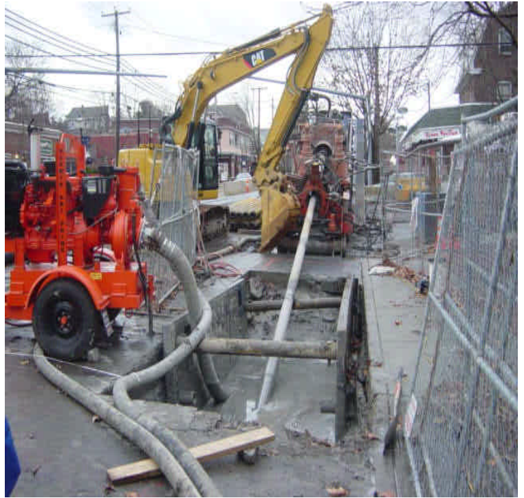
On the west side of Ash Creek, drilling continues. Adjacent catch basin remains protected. Slurry spills are common during active work but contractors state that the area is cleaned regularly.
