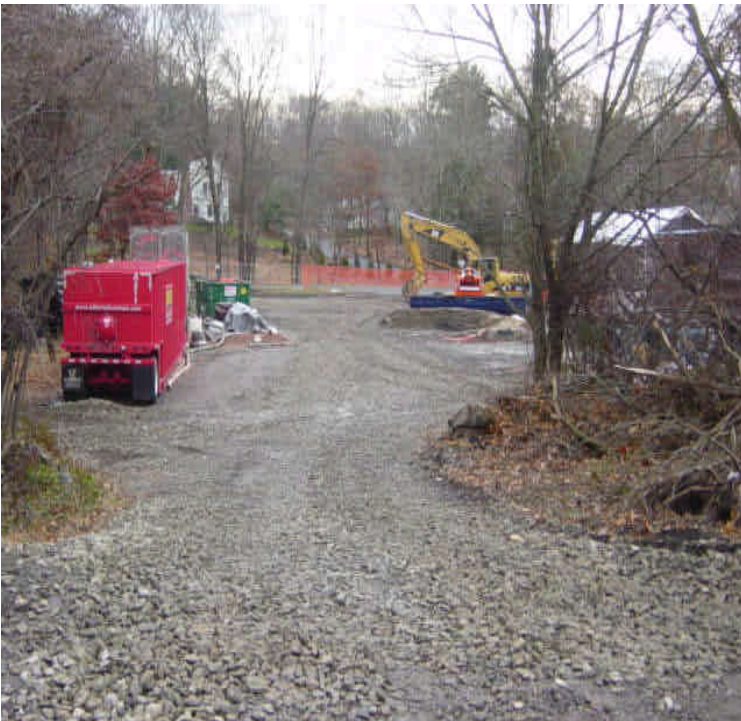
Crushed stone has been placed over the staging area on the east side of the Saugatuck River to reduce sediment tracking
