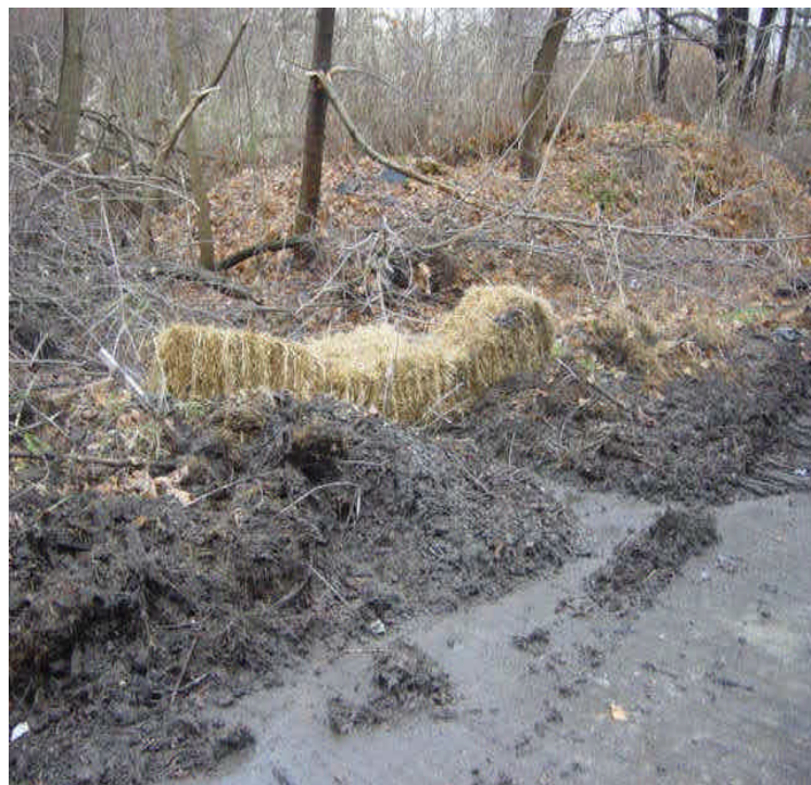
On the east side of the Housatonic River, a hay bale barrier has installed to trap sediment before it reaches the adjacent resource area. Controls should be extended to contain all exposed soil.
