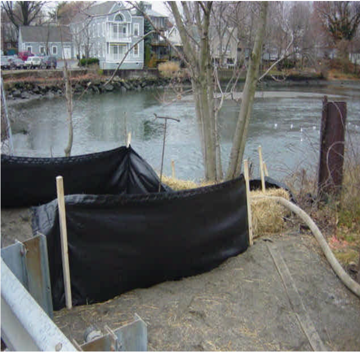
On the east side of Ash Creek silt fence and hay bales remain to prevent sediment from entering the creek near the water valve.
