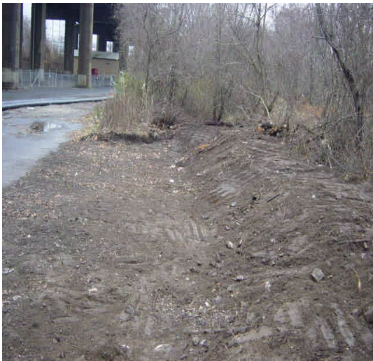
On the east side of the Housatonic River, a dirt berm has been re-graded and has been pushed closer to the wetlands. No silt fence or hay bales were observed between the exposed soil and the wetlands. Stabilize exposed soils and add controls.
