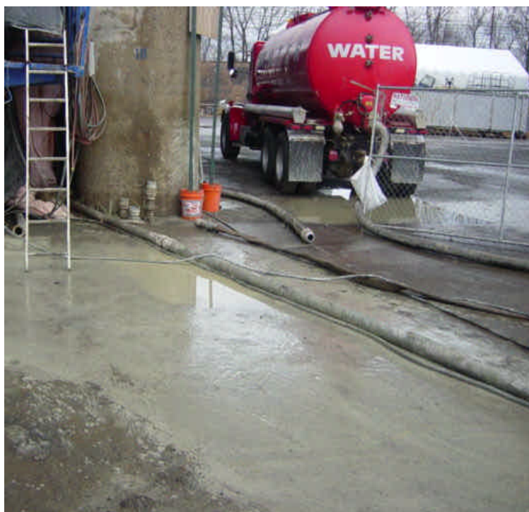
On the west side of the Housatonic River some drilling slurry has been spilled on the pavement when various hoses were disconnected. The spill was cleaned up and only residual material remained.
