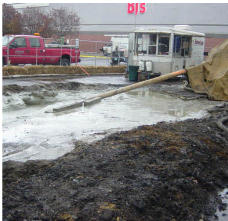
On the west side of the Housatonic River, the dirt berm around the drilling pit has been built-up and appears to be slightly higher than during the previous inspection. Slurry levels and capacity of the pit need to be monitored carefully.
