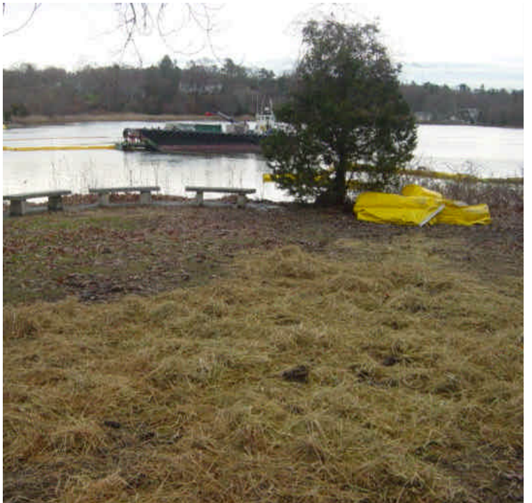
Hay mulch has been spread over exposed soils in the park area along Riverside Avenue. In the background, clean-up efforts from several drilling frac-outs continue along the Saugatuck River.
