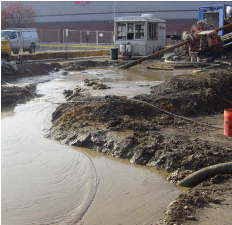
Drilling pits on the west side of the Housatonic River have a small dirt/sand berm around portions of the perimeter. Drilling fluid/mud is less than 6" from overtopping the drilling pit in some locations. Ensure that capacity is adequate.
