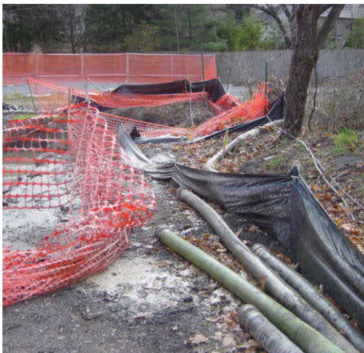
The silt fence around the drilling pit on the east side of the Saugatuck River is sagging and needs attention. Drilling fluid splashed beyond the contained limits of the silt fence.
