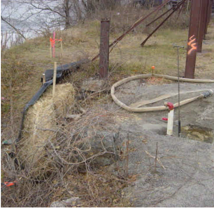
The small area of soil excavated on the northeast side of Ash Creek near the water valve has been contained with silt fence and haybales to minimize the potential for sediment entering the creek.
