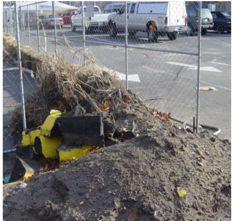
On the west side of the Housatonic River, excavated asphalt, soil, and other debris has been temporarily stockpiled at the perimeter haybales containing the work zone. Pull the material back to ensure the controls remain effective.
