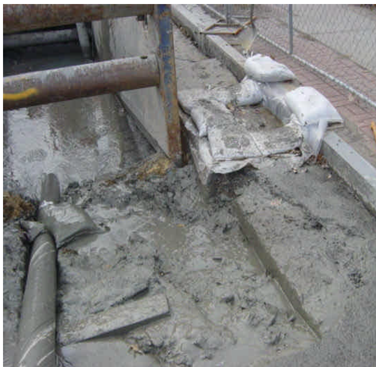
A significant amount of drilling slurry has spilled on the pavement on the east side of Ash Creek near the drilling pit. Although the catch basin has been protected, sweep and remove the material.
