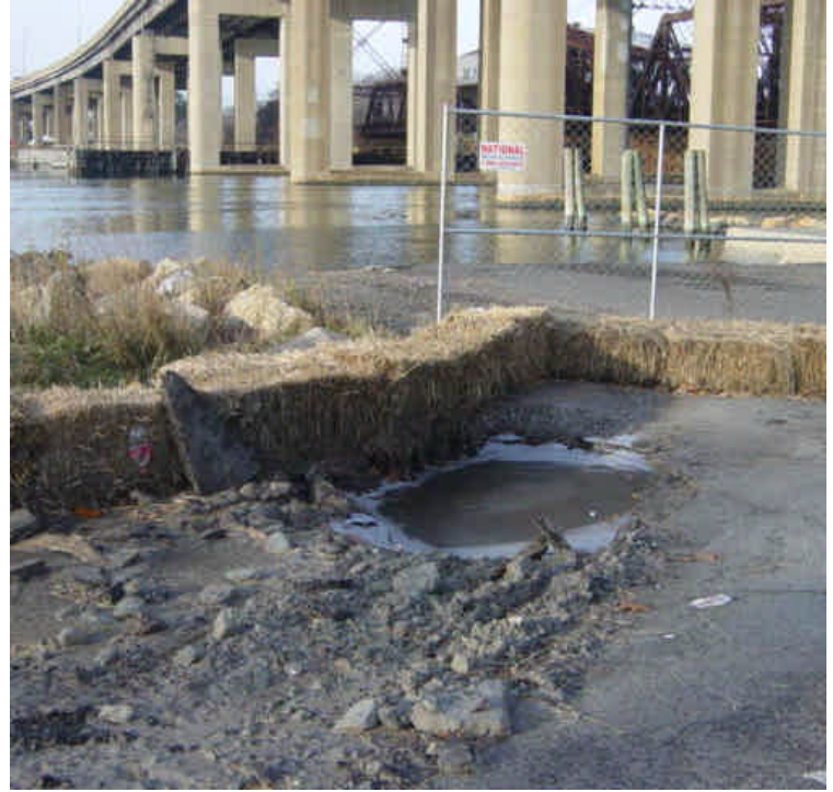
On the east side of the Housatonic River, holes formed in the pavement due to pressure from the HDD operation (similar to a frac out). Crews excavated the area and used a vac truck to remove any remaining material. Haybales were placed around the area to provide additional containment.
