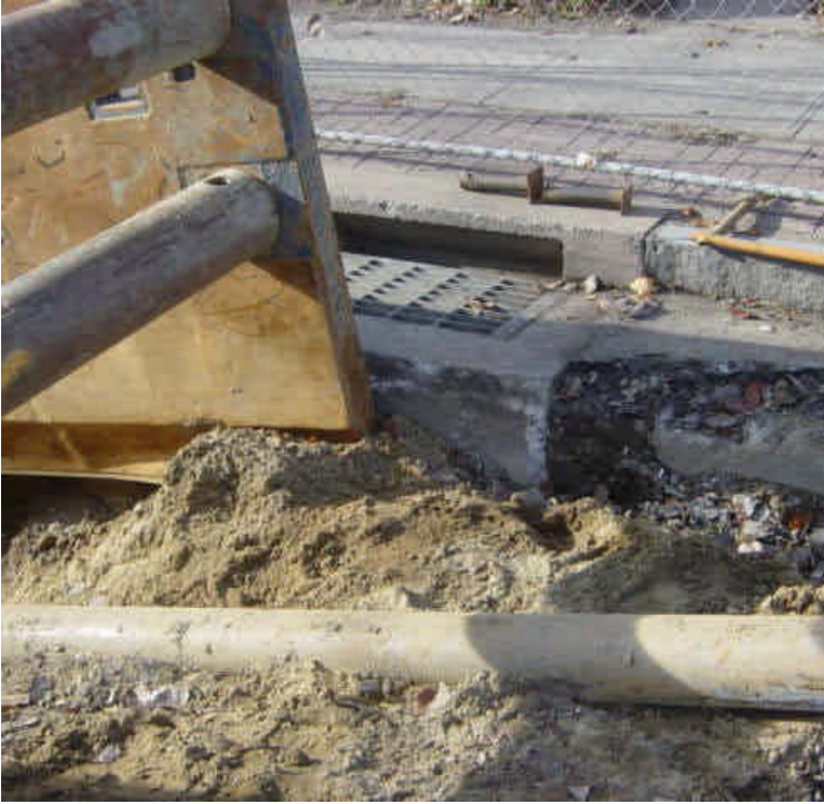
Horizontal directional drilling (HDD) continues near Ash Creek. A drilling pit has been excavated on the northeast side of the creek. A catch basin adjacent to the drilling pit is not protected.
