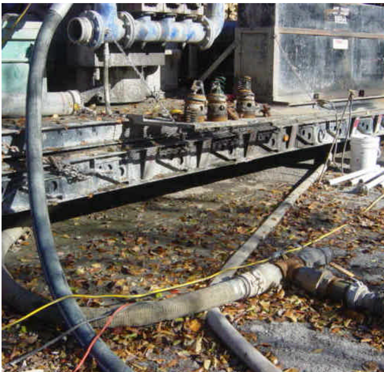
Slurry residue/drilling mud spills remain in several locations in the staging area on the east side of the Saugatuck River. Slurry spills were observed in multiple locations behind the bentonite reclamation machine and near the drilling pit.
