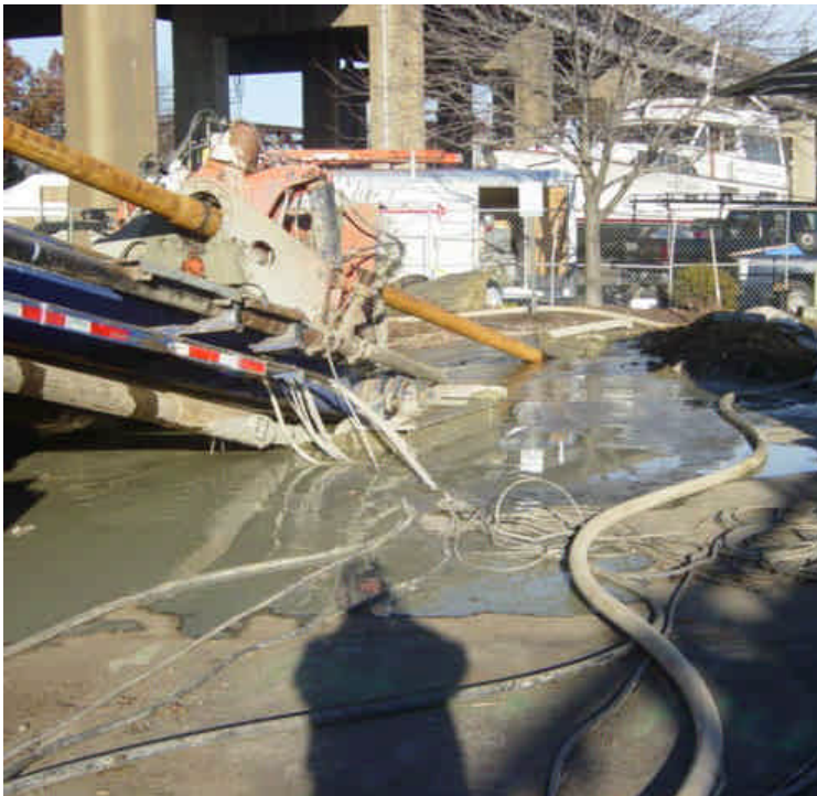
HDD is underway on the west side of the Housatonic River. The drilling pit appears to be adequately sized, but has been located several feet from where the drill string is actually entering the ground. Slurry material is not being aimed directly into the drilling pit and is flowing over the paved area. Perimeter controls are in place around the staging area, but slurry material should be better contained to minimize unnecessary impacts.
