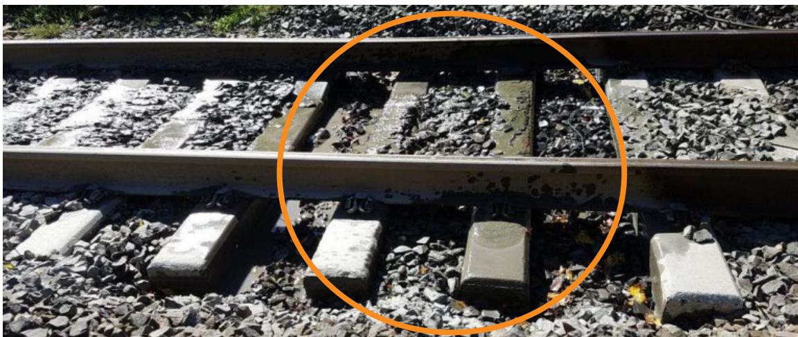
Figure 2 Concrete Tie Damaged Due to Poor Drainage
