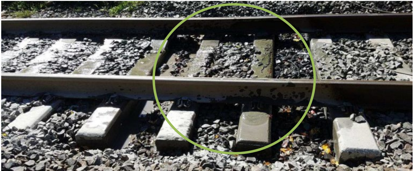
Figure 11: Example of Fouled Ballast Resultant from Poor Track Drainage
