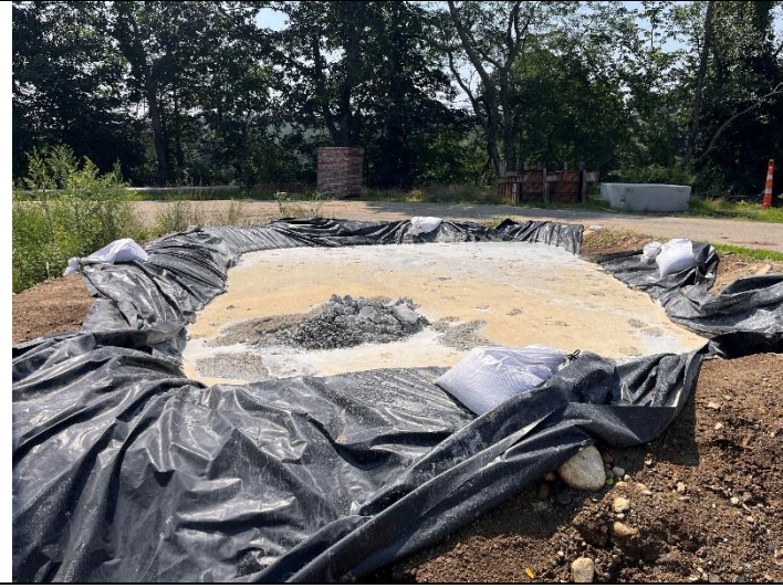
Concrete clean-out should be contained for proper disposal. See example above.
