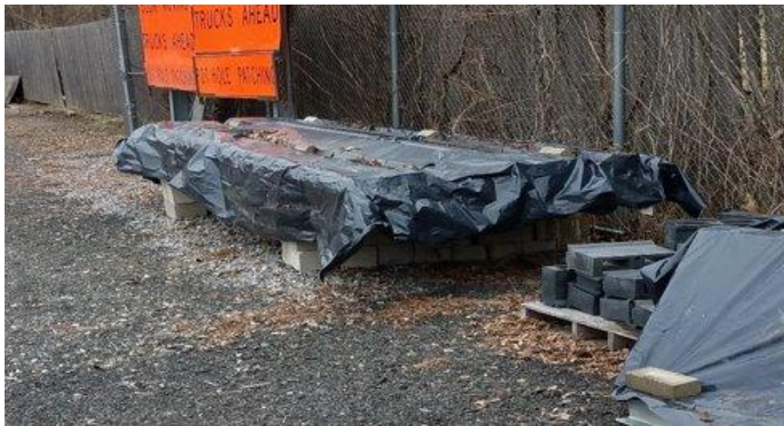
Elevate and cover galvanized steel with tarps to the extent possible. See example above.
