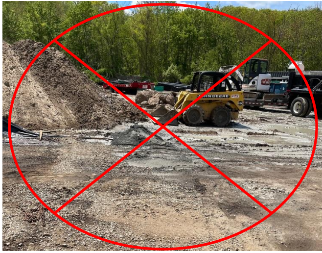
Concrete clean-out should be contained for proper disposal. See example above.
