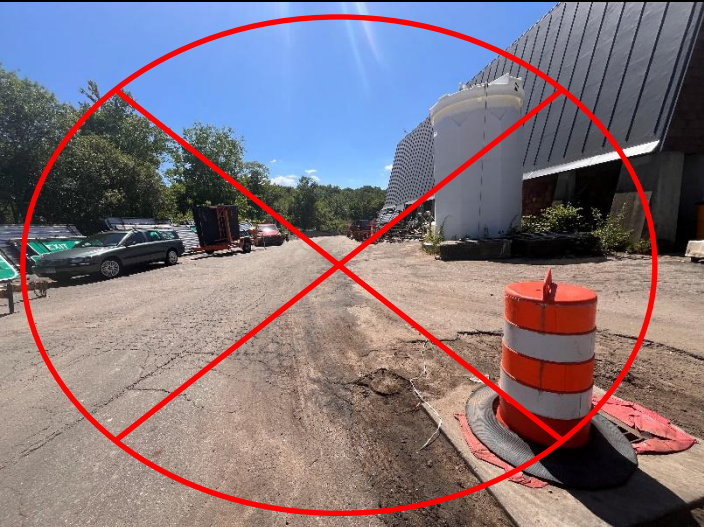
Maintain pavement around catch basins.
