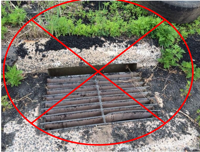
Loose material should not be stored around catch basins.
