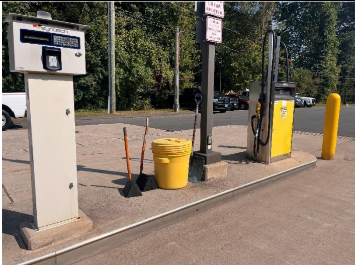
Keep spill kits and catch basin covers available near fueling and petroleum storage areas.
