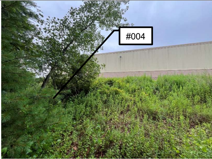
Outfall #004 located on the west of the Site. 15" RCP at the toe of the slope behind the Bridge Building.
