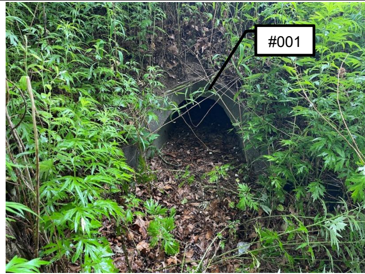
Outfall #001 located on the west of the Site. 15" RCP at the toe of the slope behind the Bridge Building.
