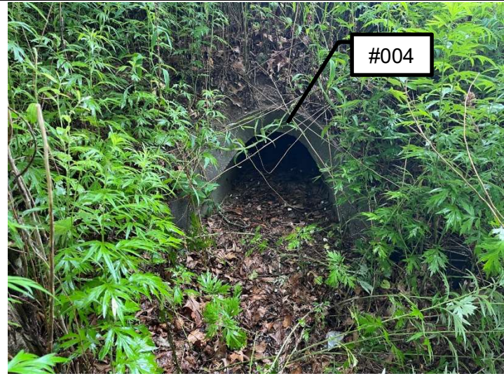
Outfall #004 located on the west of the Site. 15" RCP at the toe of the slope behind the Bridge Building.
