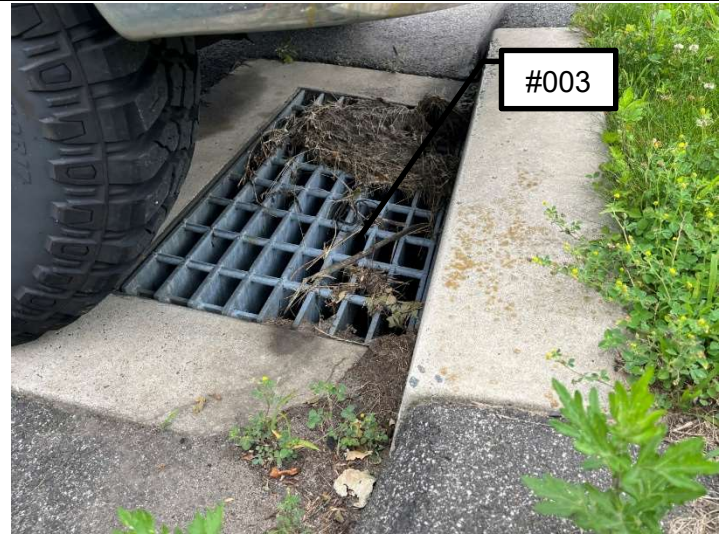
Outfall #003 located on the east of the Site. Outlet pipe within the catch basin structure is Outfall #003.
