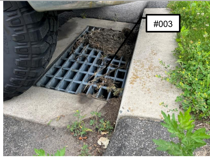
Outfall #003 located on the east of the Site. Outlet pipe within the catch basin structure is Outfall #003.
