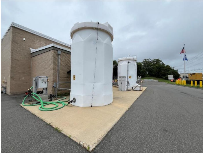
Keep area around magnesium chloride tank free from parked vehicles and stored material to the extent possible. (Additional magnesium chloride tank added, see photo at end of table)
