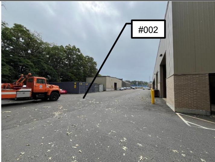
Outfall #002 located on the northeast of the Site. Outlet pipe within the manhole structure is Outfall #002.
