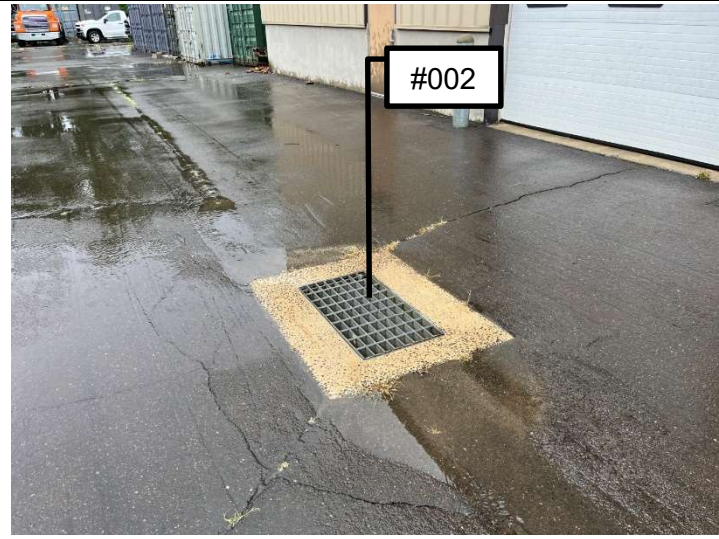
Outfall #002 located on the northeast of the Site. Outlet pipe within the catch basin structure is Outfall #002.
