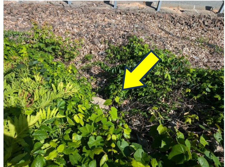
Outfall #002: Flared outfall to swale on south side of the entrance drive (clearing of vegetation required)
