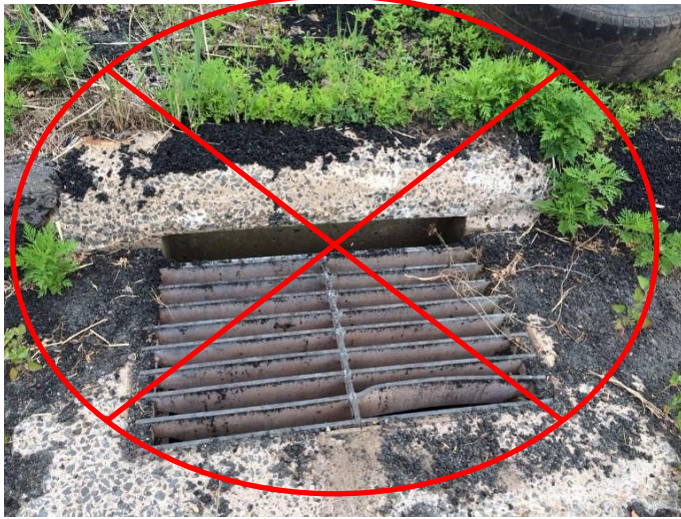
Loose material should not be stored around catch basins.
