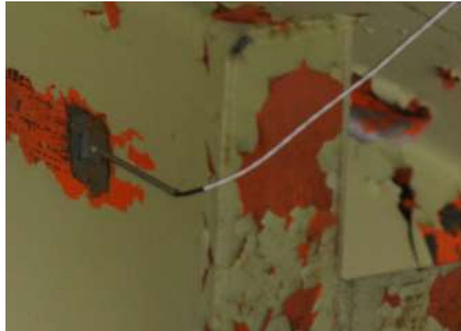
Figure 30: An installed resistance temperature detector on the Meriden Bridge
