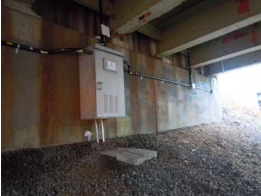
Figure 17: Cabinet housing system components under Meriden Bridge
