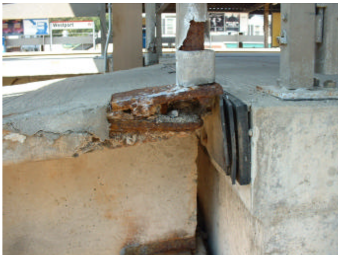
Ramp Corrosion and Spall
