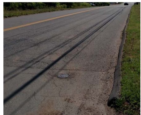
Figure 7. No Shoulder Lines
