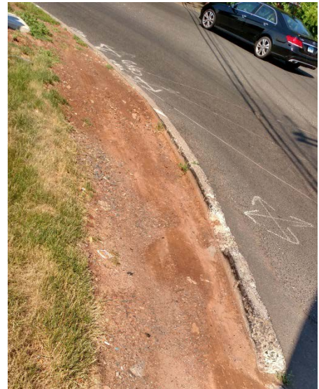
Figure 5. Tire Track Marks Going Over the Curb
