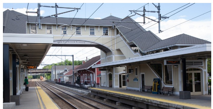
Figure ES-8: Railroad electrification infrastructure at Old Saybrook Station
