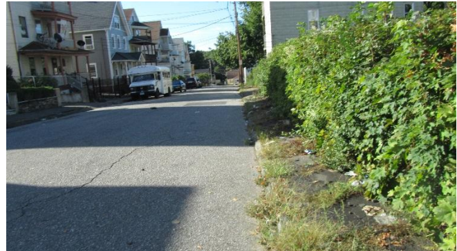
Figure 12: Deteriorated Sidewalk on South Street
