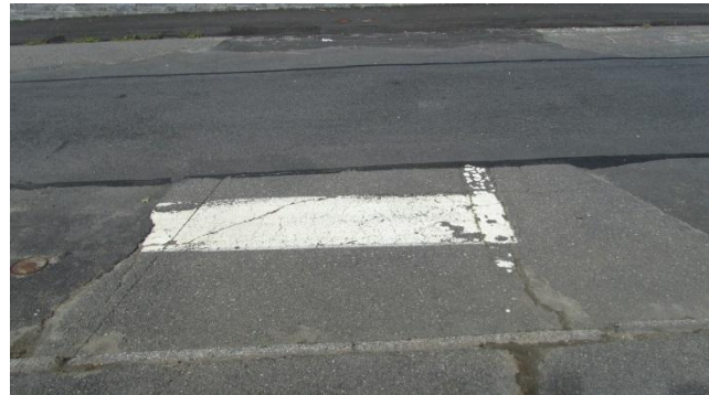
Figure 19: Crosswalk Paved Over on Xavier Street
