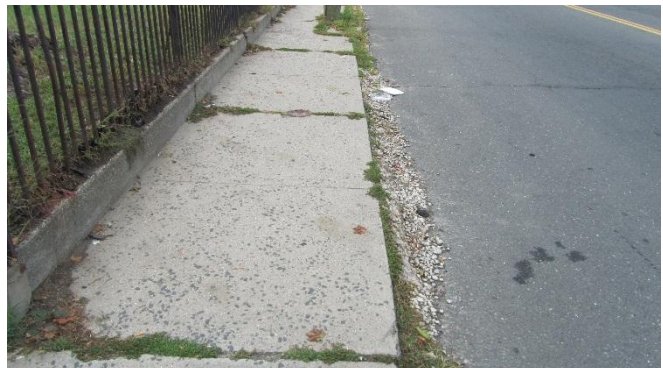
Figure 16: Completely deteriorated curb along Baldwin Street
