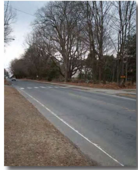
View of crosswalk on Cross Street. Crosswalk is hardly visible given lack of signage.
