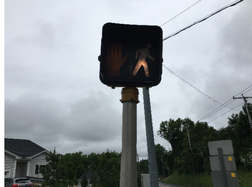
Figure 26: Pedestrian Beacon at Tryon Street and Saybrook Road
