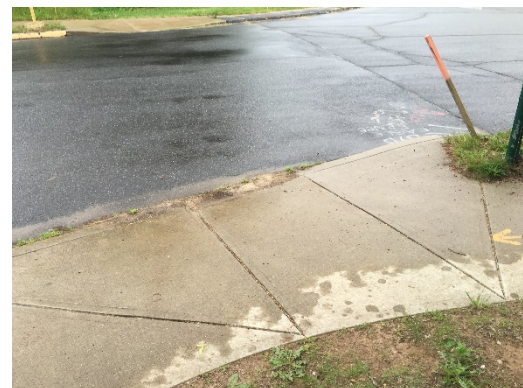
Figure 30: Current Non-ADA Compliant Ramp
