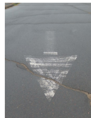
Figure 4: Faded Pavement Marking in School Lot
