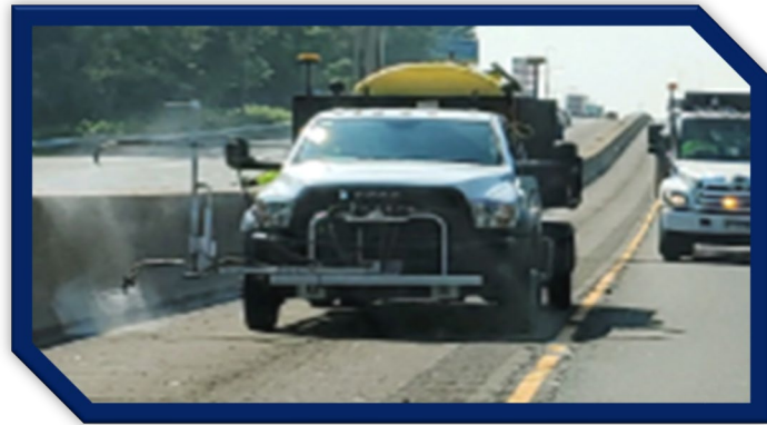
Herbicide application is necessary along structures such as median dividers where mowing is impractical.
